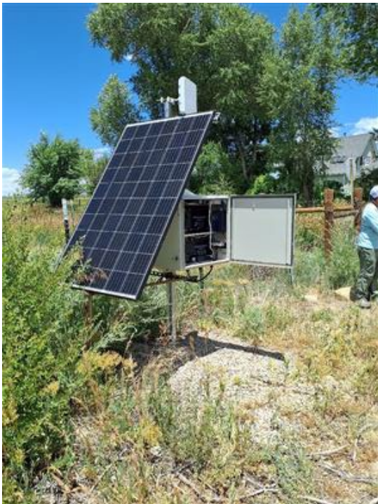
Photo 3. Typical Telemetry Installation
