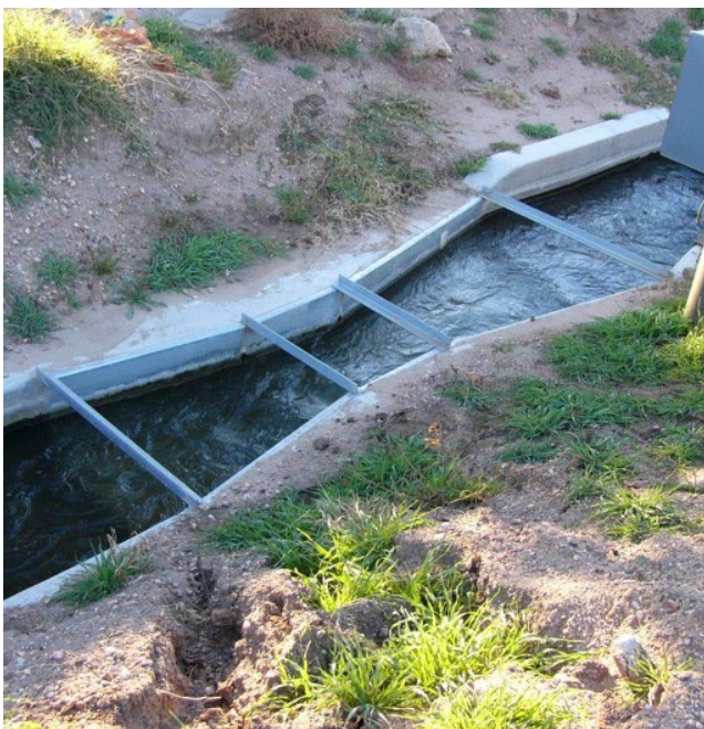
Photo 1. Typical Parshall flume installation
