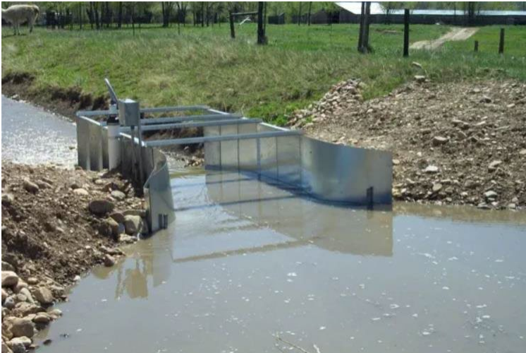
Photo 2. Typical ramp flume installation
