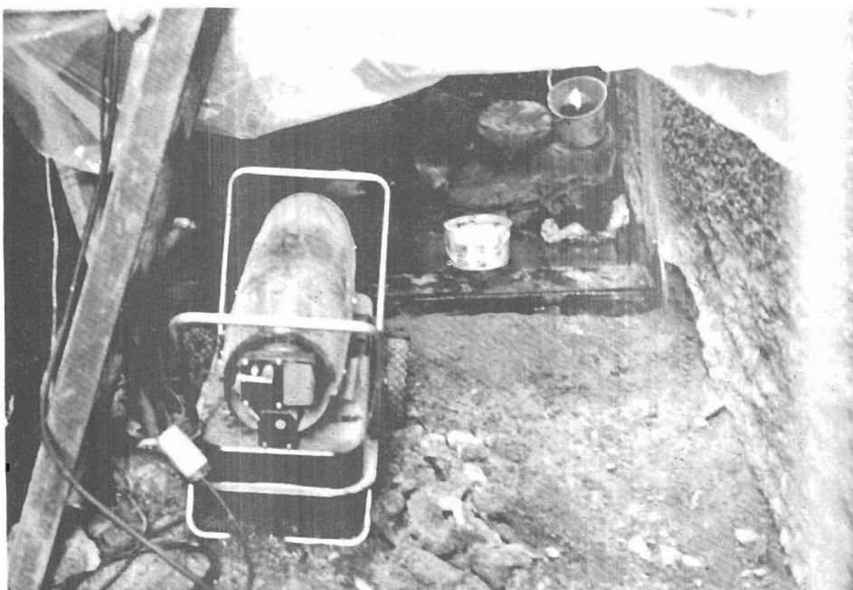
Forced air heater used for drying.
