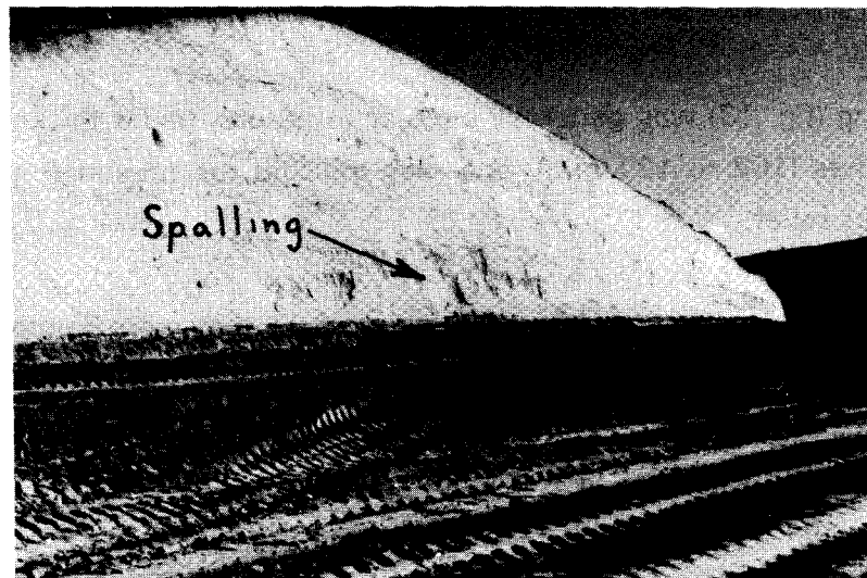
Figure 13. – Spalling on cut slope of Mirdan Canal. P801-D-81426.
