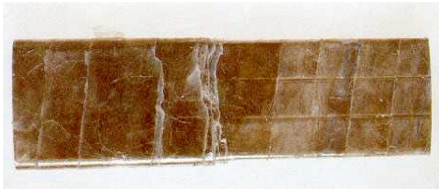
Figure 12.—Portion of unused spare coil showing normal color of binder. P801-D-79799.
