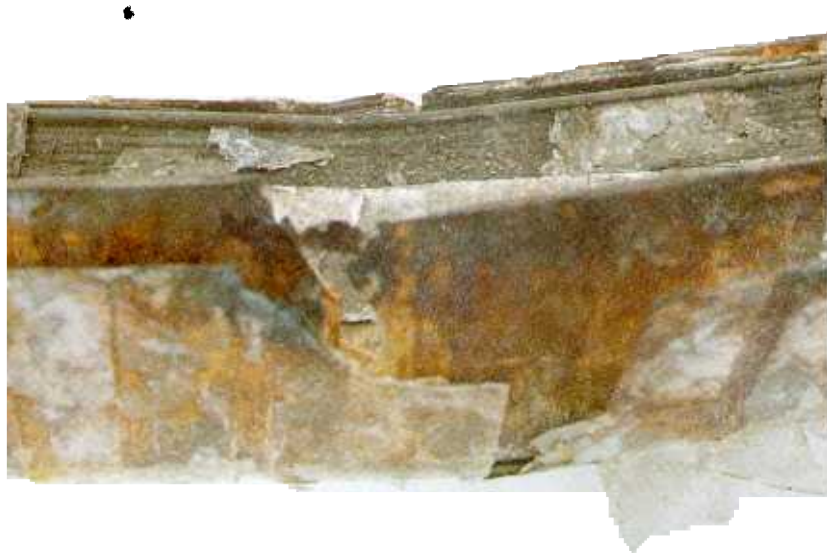
Figure 9.—Closeup view of dissected coil prior to removal of all groundwall and turn insulation P801-D-79796.
