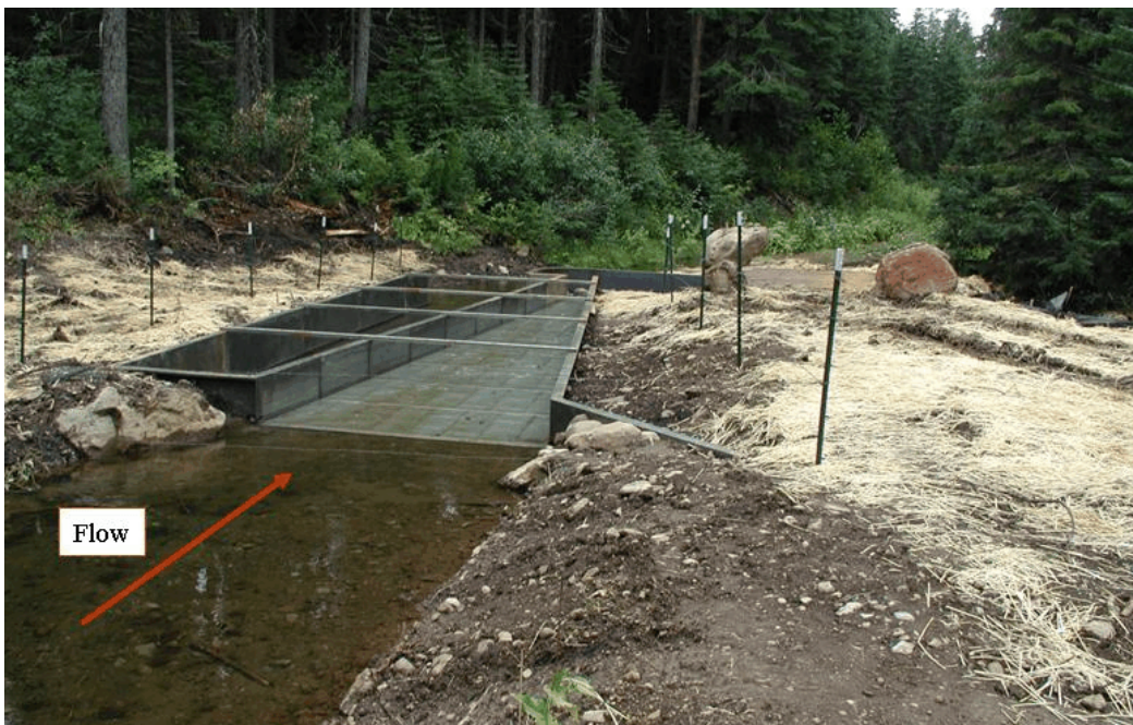
Figure 20.—Horizontal flat plate screen, East Fork Ditch Company, East Fork, Weiser River, Idaho.
