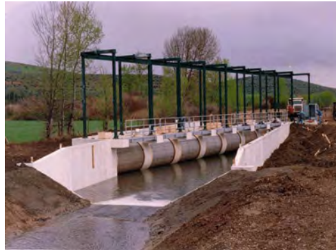
b. Cascade Canal fish screen monorail hoist.
