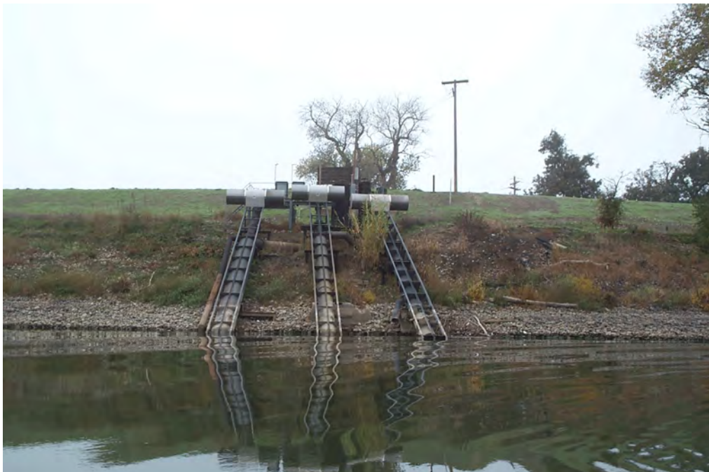
Figure 16.—Installation showing three raised retrievable cylinder screens – Davis Ranches Site #1, California (intake screens incorporated).
