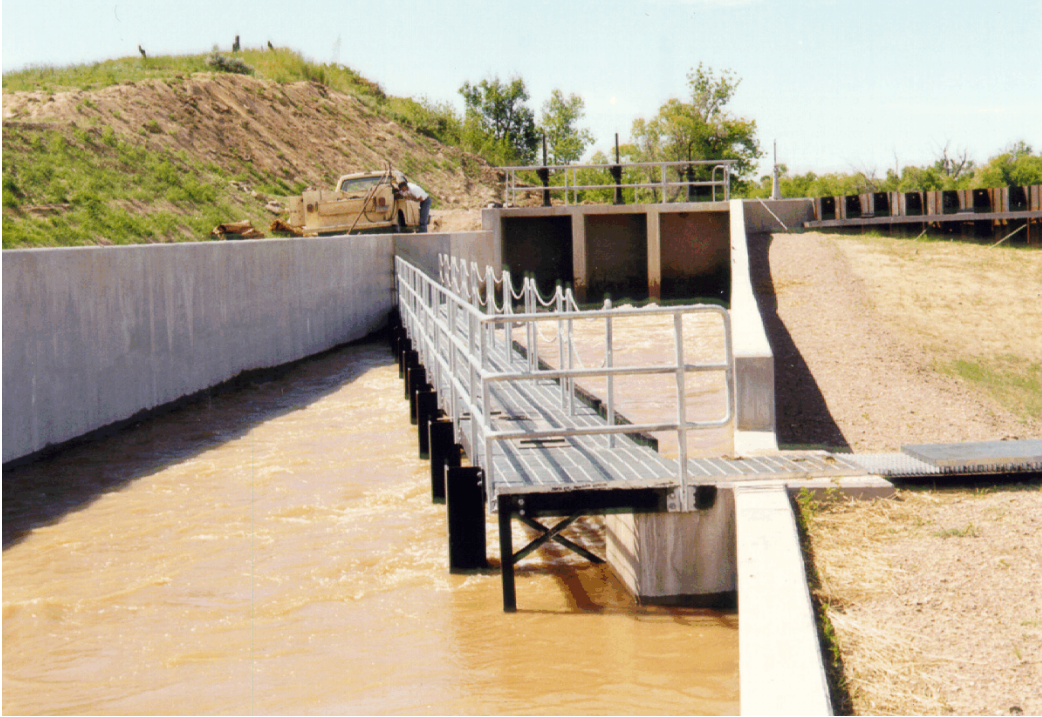
Figure 119.—View looking upstream at the T&Y louver placed at an angle to the canal flow – Example 4 (T&Y Irrigation District).
