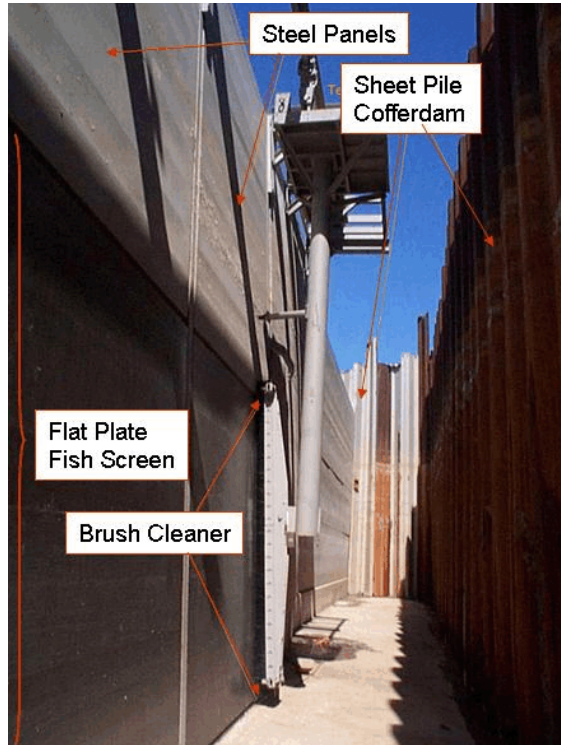
Figure 64.—Flat plate screens with horizontal brush cleaner (GCID).
