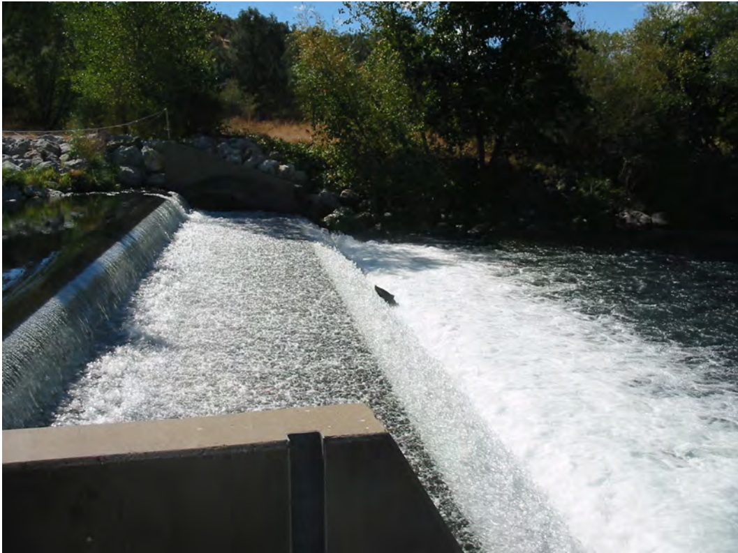
Figure 127.—Fish barrier weir at Coleman National Fish Hatchery, Battle Creek, California.
