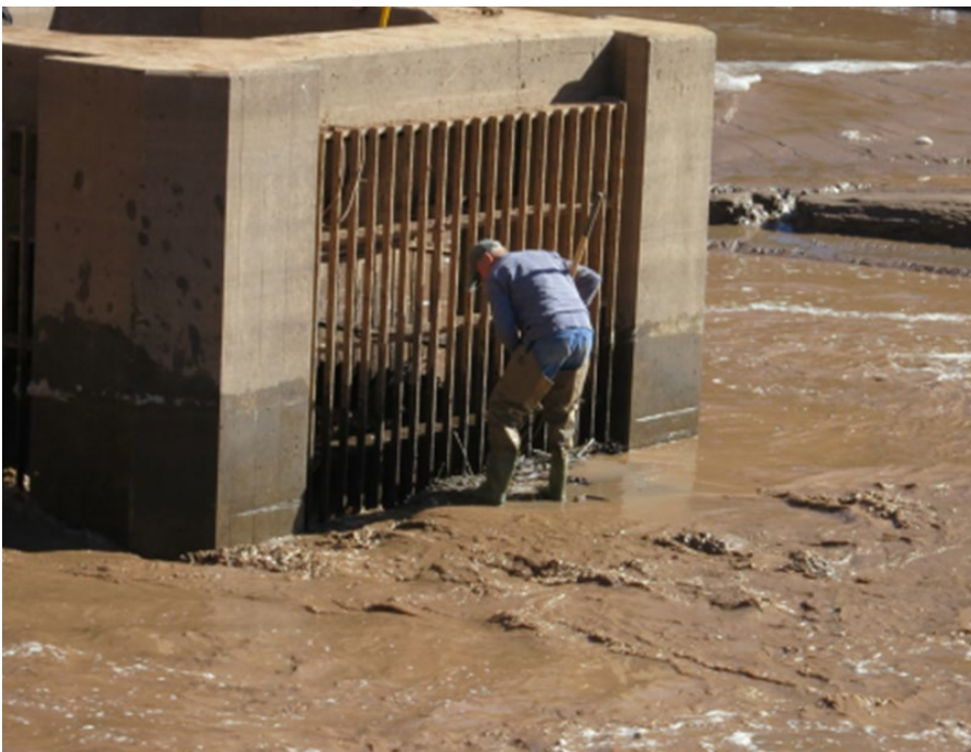
Figure 10. Paonia Dam outlet structure during emergency actions to maintain diversion, Bureau of Reclamation photo Nov 11, 2014.
