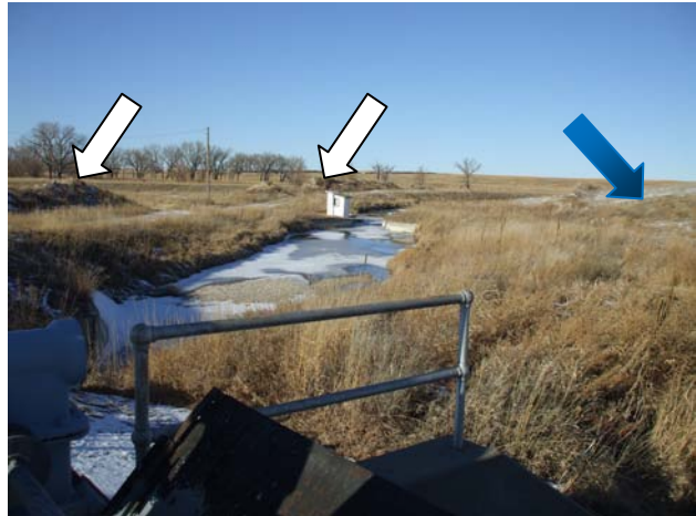
Figure 7. Parshall Flume below Dunlap Dam
