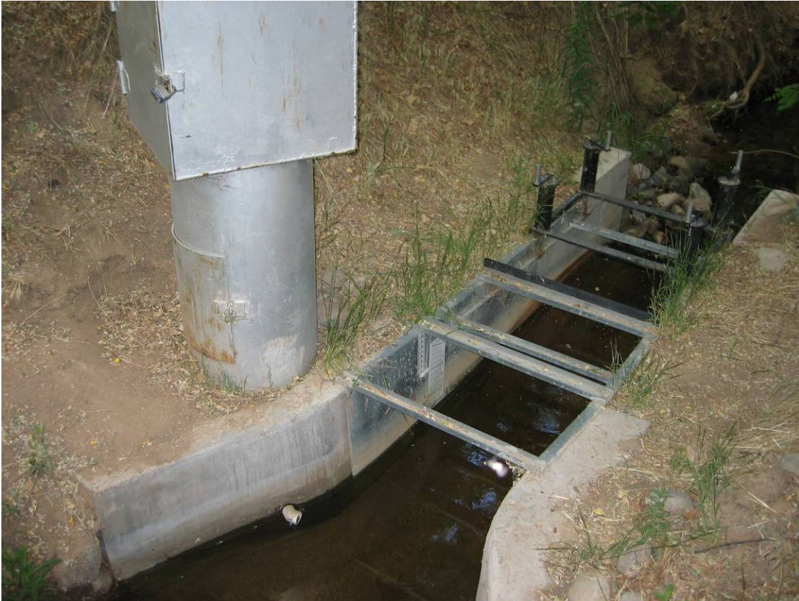
Figure 5—improper stilling well inlet location, elevation, and configuration.
