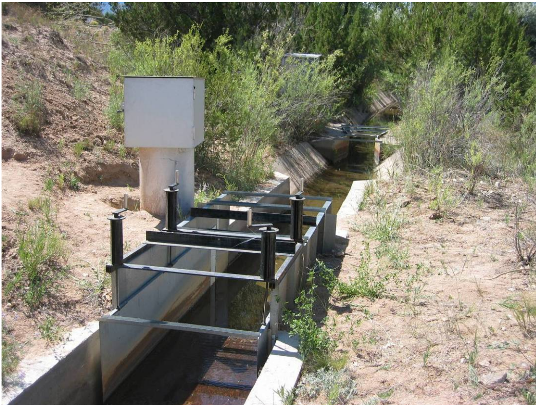
Figure 2—Adjust-A-Flume™ ramp flume with stilling well and equipment shelter. Note the abandoned Parshall flume located upstream.
