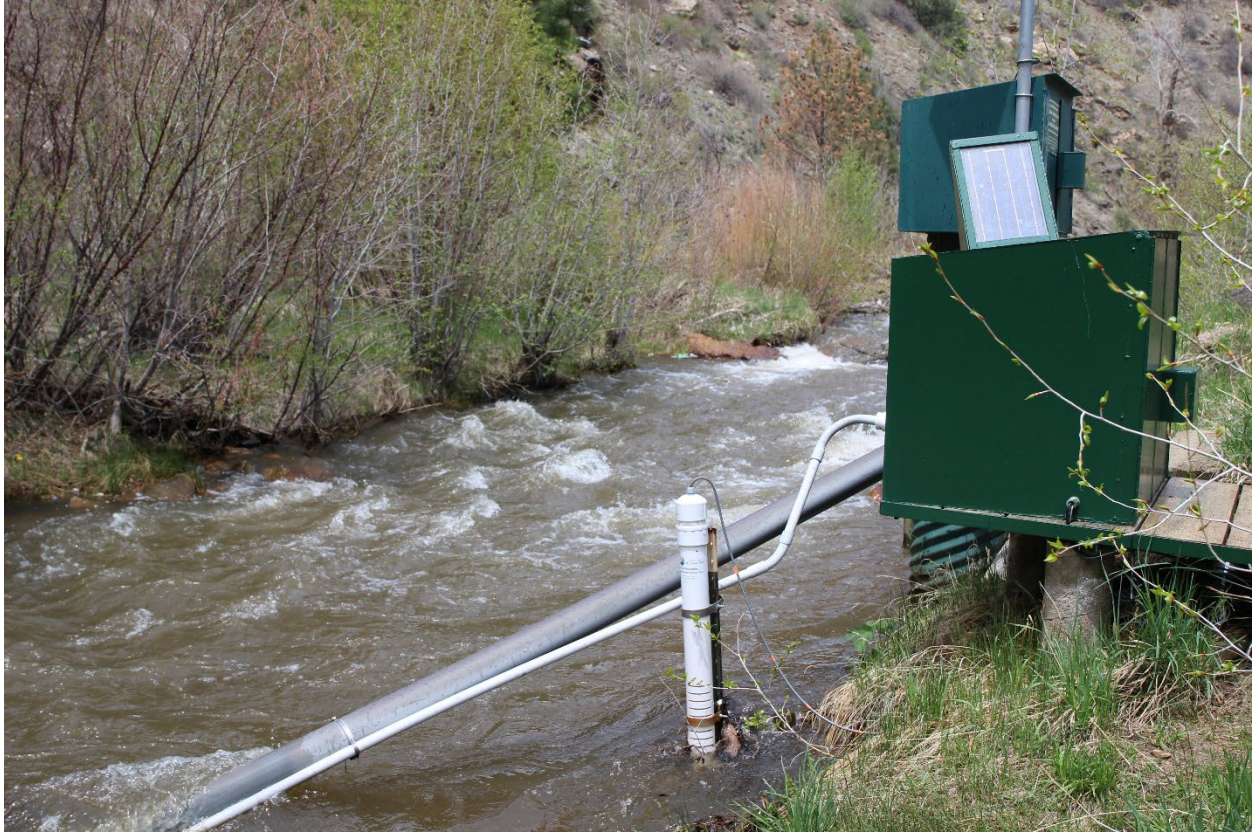
Figure 11 – Photograph showing the eTape® sensor installed at the Clear Creek location.
