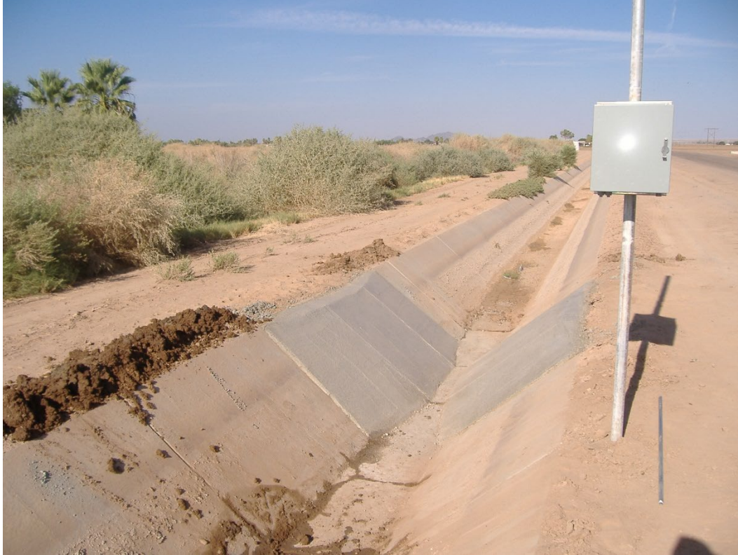
Figure 6. Pueblo canal long-throated flume pictured shortly after its construction in 2019.
