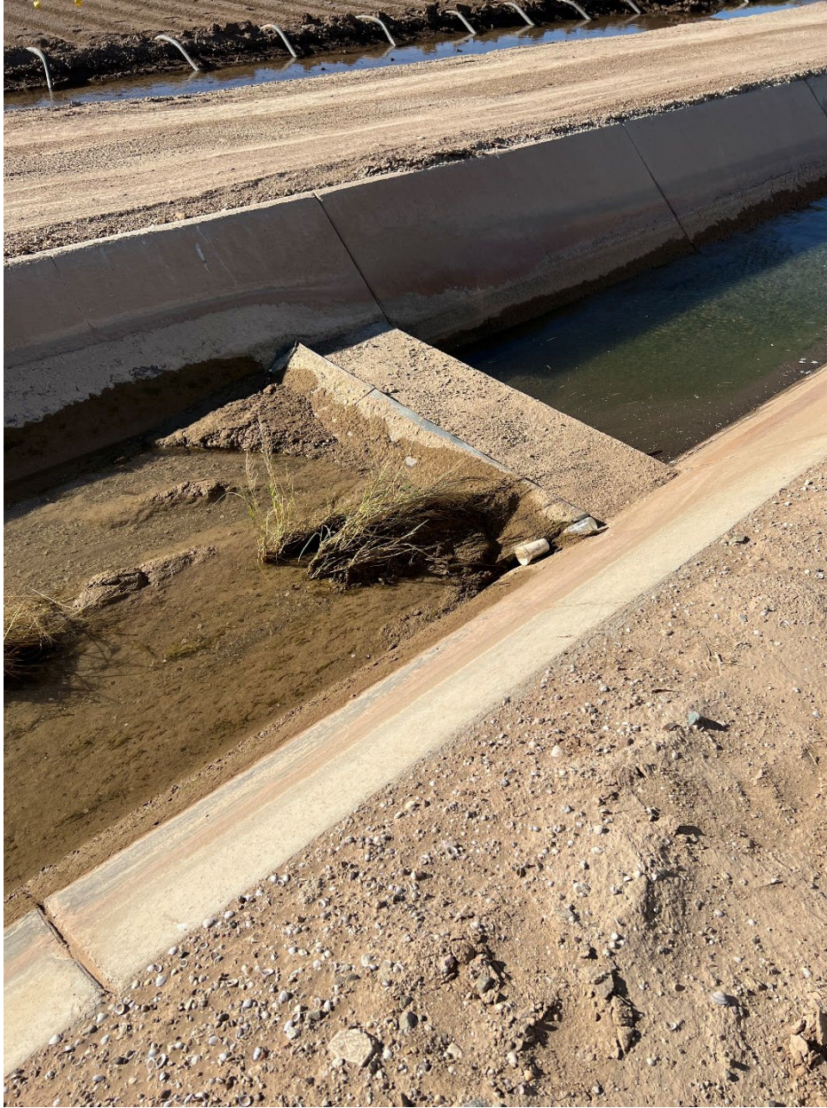
Figure 5. Supai canal ramp flume pictured during a 2022 site visit showing excessive sediment with vegetation against the ramp of the flume.
