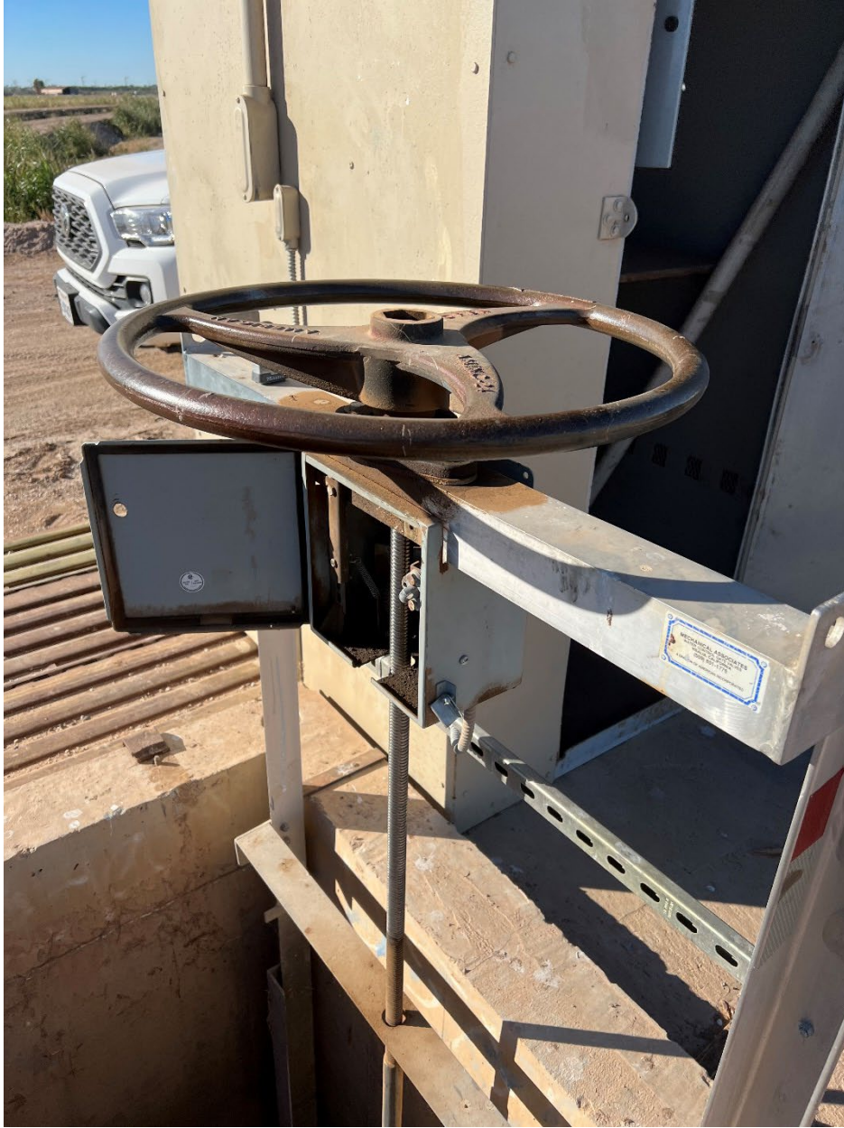
Figure 2. Manually operated 36-inch slide gate at the Waco Diversion Structure.
