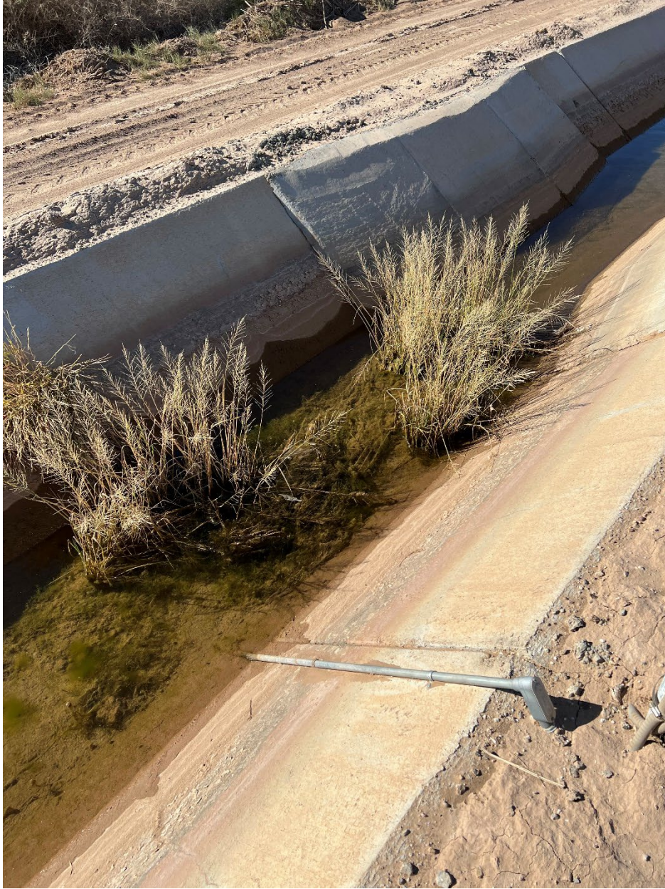
Figure 7. Pueblo canal long-throated flume pictured during a site visit in 2022 showing excessive sediment and vegetation upstream of the flume.
