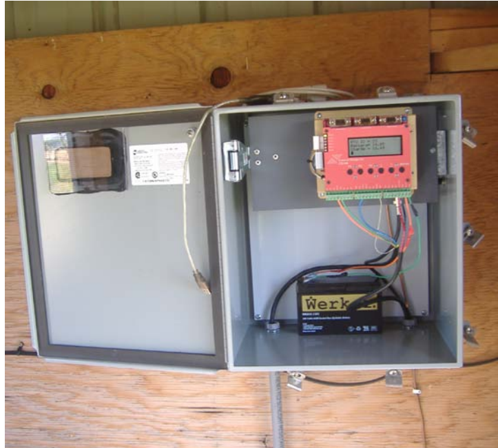
Figure 6. A CDI Radio/Control Unit Installed in the Pump House Shown in Figure 5
