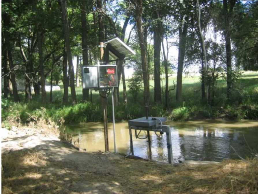
Figure 7. Gate Automation Equipment at SPDC Company Lateral Headgate
