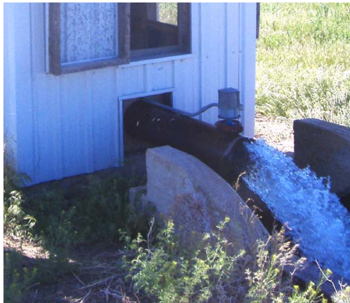
Figure 5. A Pulse Output Module Installed on a McCrometer Meter at a J & E Well
