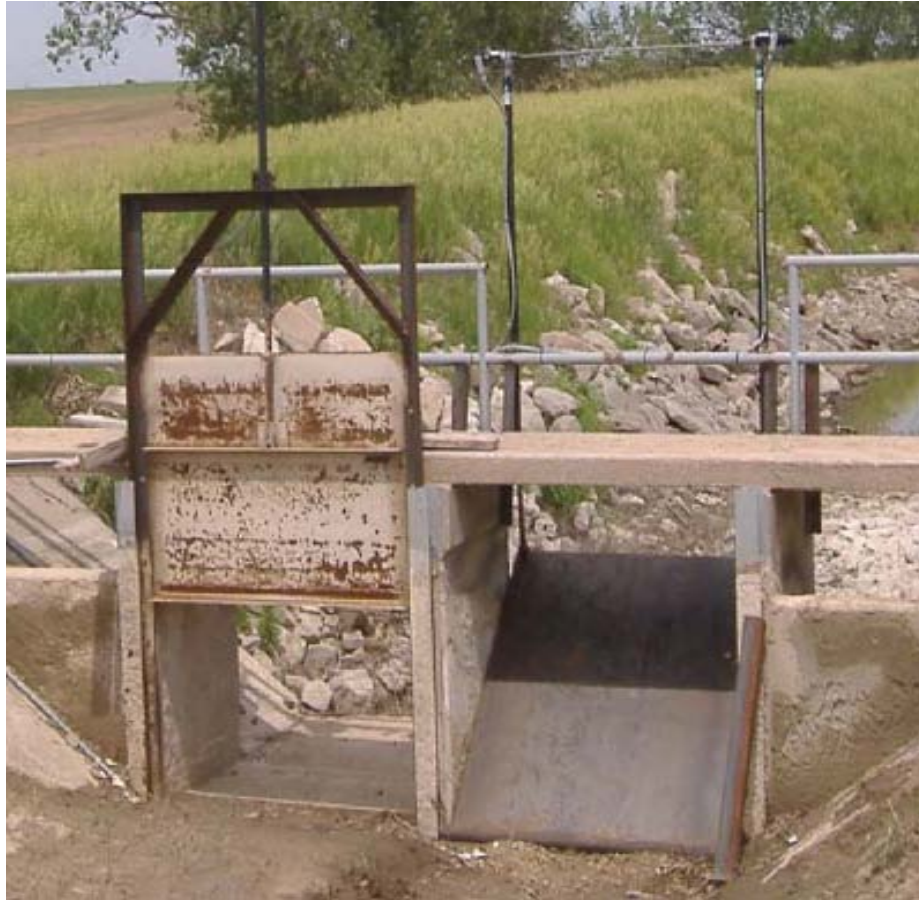
Figure 7. Vertical Slide and Overshot Gates at the 28.6 Check Both Motorized using DC Linear Actuators
