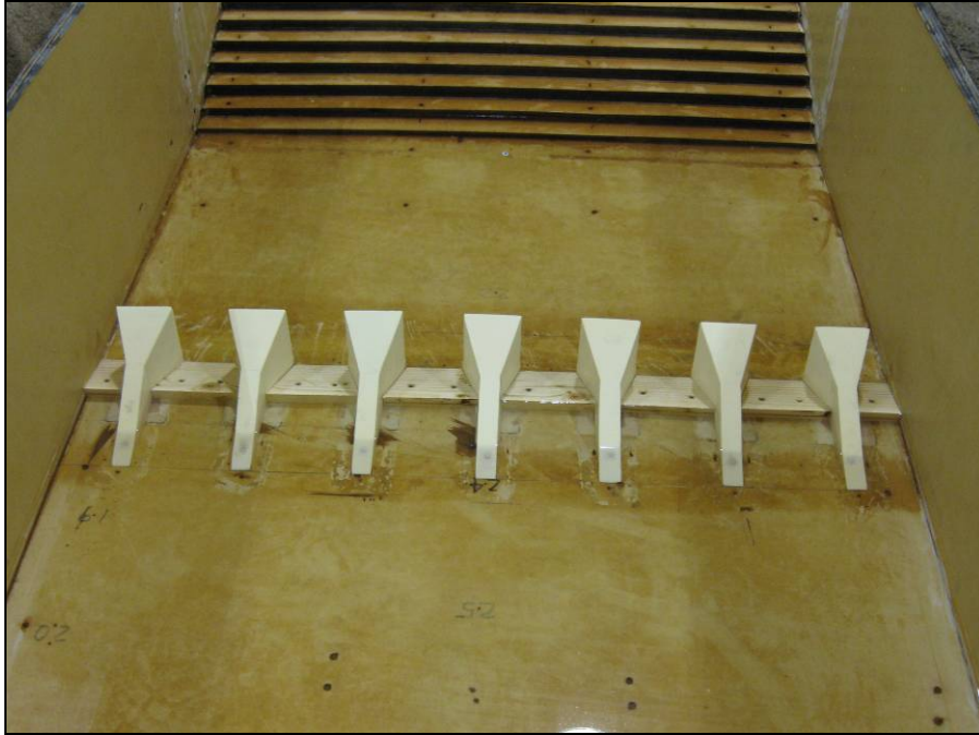
Figure 7. Looking upstream at the cavitation-reducing baffle blocks with a 4-ft-high by 12-ft-long ramp on a 3:1 slope between the blocks.
