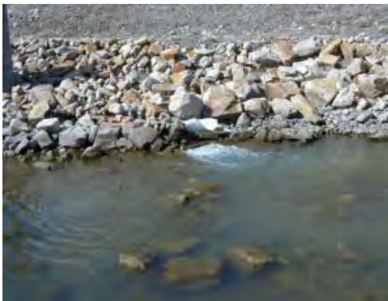
Figure 4. - Close up view of the bypass pipe exit. A standpipe is located on the very left side of the picture. The standpipe was installed to allow air to escape from the flow.
