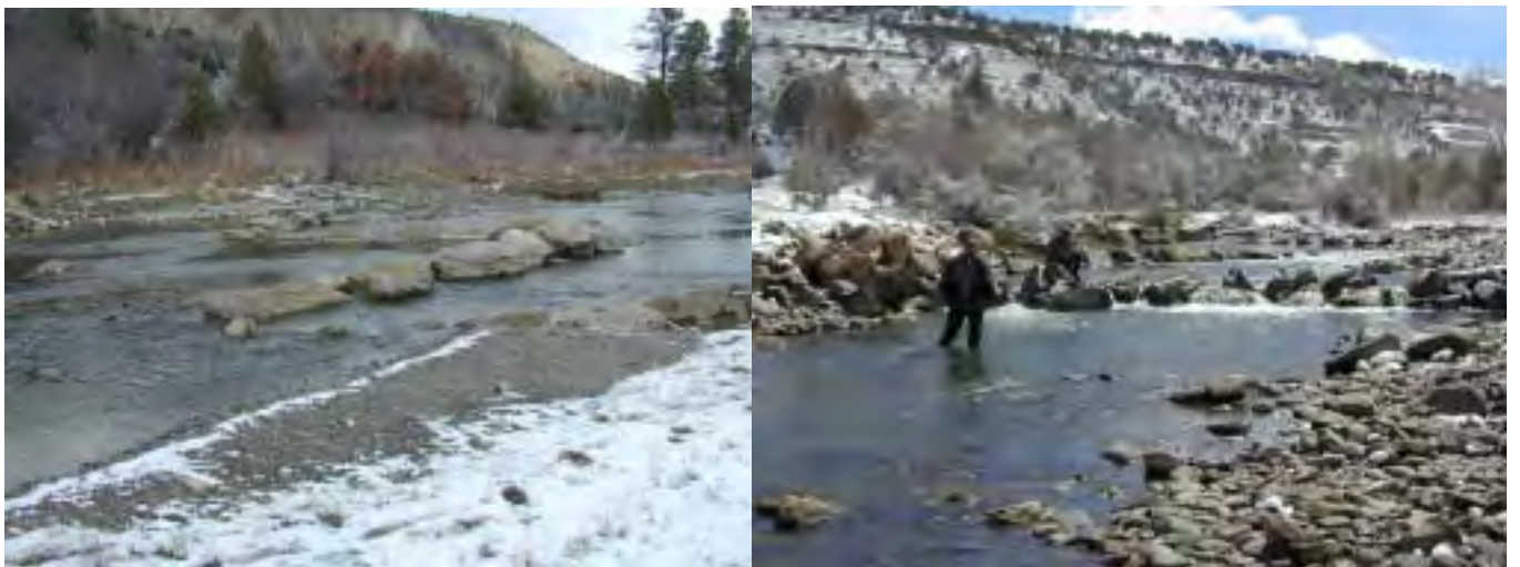
Figure 10. - Example of two rock weirs or Rosgen habitat structures that have been installed in the stream below Ridgway Dam to provide habitat and help improve water quality.
