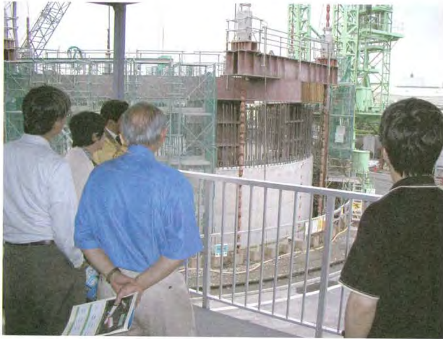
Vertical Shaft, The Metropolitan Area Outer Discharge Channel, Chiba, July 18, 2003
