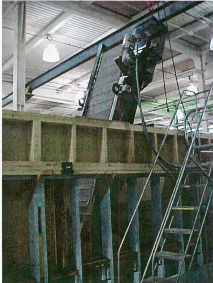
Figure 1. Traveling water screen installed in test flume at 70 degrees.
