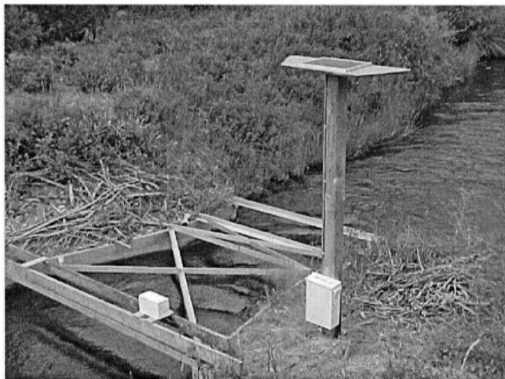
Figure 5. Continuous flow meter (CFM) installed on a Parshall Flume at Dillon Montana.
