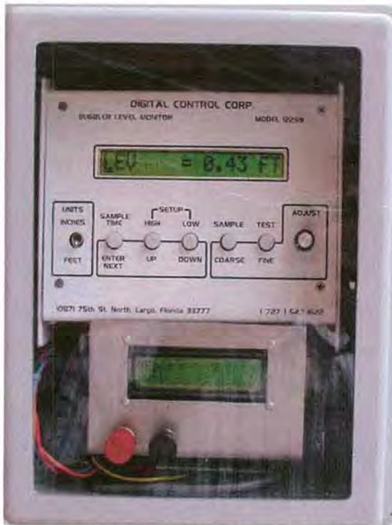
Figure 3. - Close up of the bubbler electronics on top and the OCFR electronics on the bottom. This allows totalizing of the flow from the bubbler water level information.
