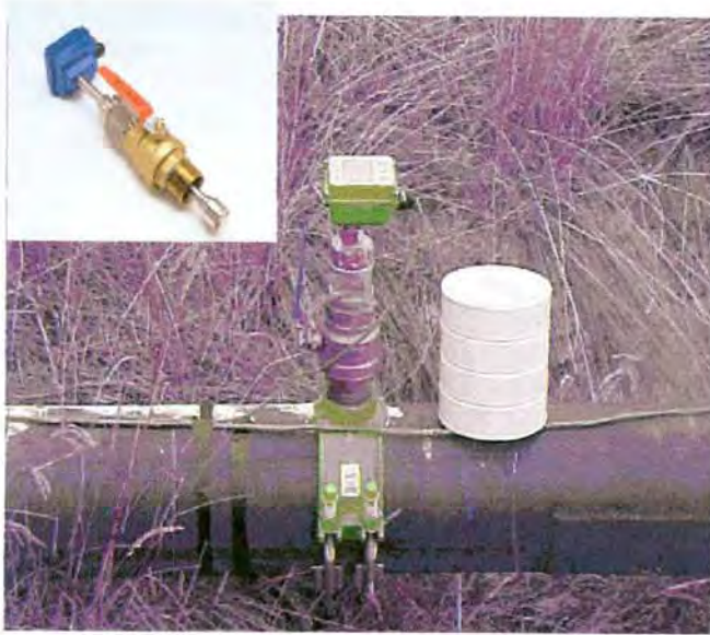
Figure 6. - SeaMetrics paddle wheel flow meter with display installed on an 8 in pipe in Montana. These meters may be used on pipes between 2 and 48 inches in diameter. (The white can is placed over the sensor to provide shade.)
