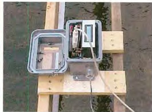
Figure 2. - View looking into the OCFR. The cable is hooked to a laptop computer for easy programming of the CPU or downloading stored data. The display shows flow in \text{ft}^3/\text{s} and total flow in acre-ft. The ultrasonic sensor is underneath the box above the water level.
