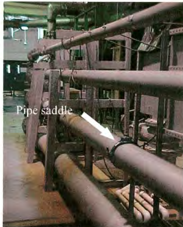
Figure 11. - WRRL pipe test stand showing the pipe saddle on the 8 in pipe where the flow meters were tested. The pipes in the stand are 4, 6, 8, and 12 inches in diameter.
