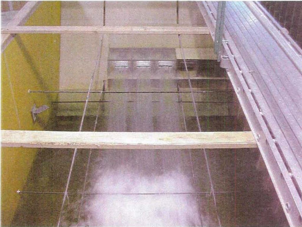
3 gates operated at 10% open in free-discharge mode.
