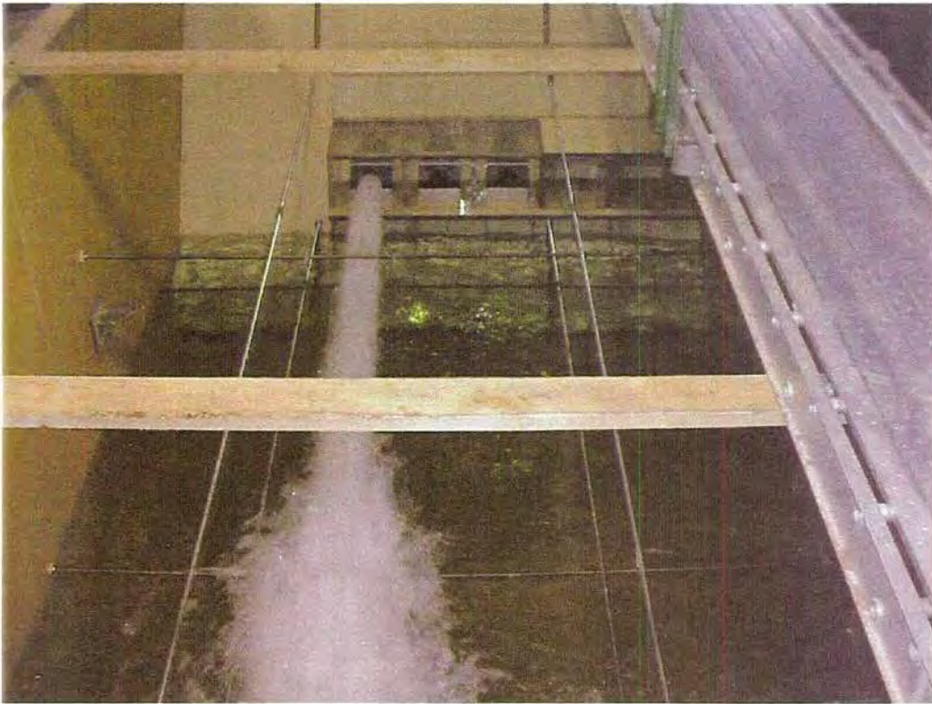
1 gate operated at 100% open in free-discharge mode.
