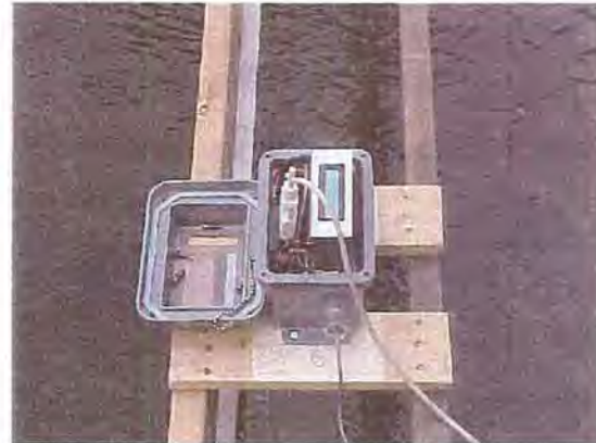
Figure 10 - Self-contained ultrasonic flow measurement recorder and data logger.
