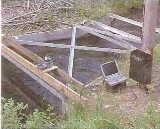
Figure 9 - Parshall Flume at East Bench
