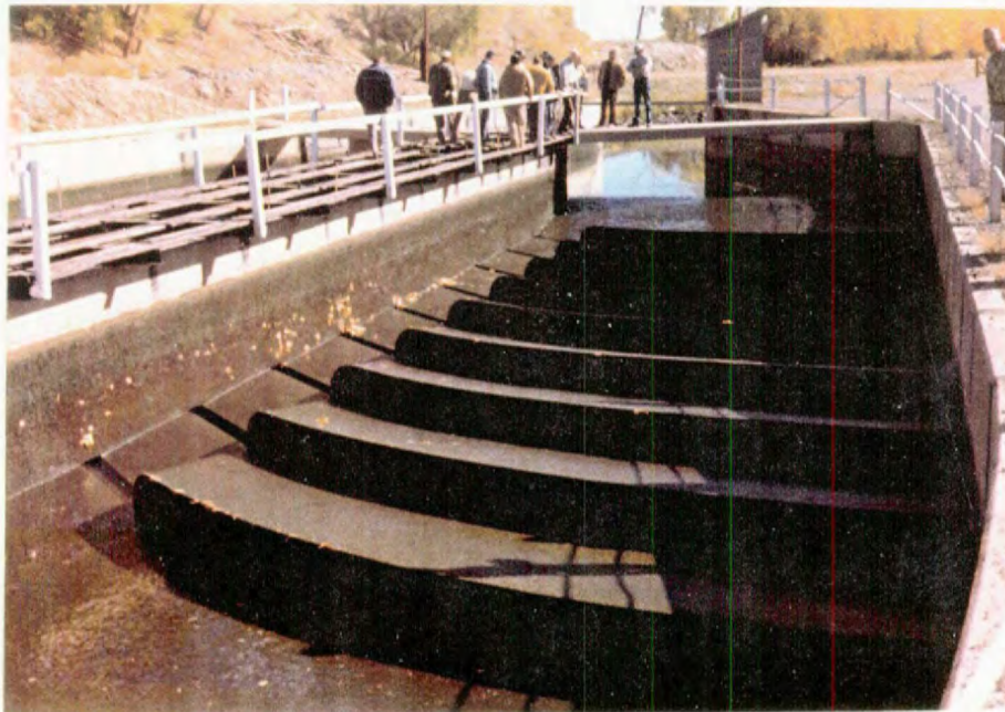
Downstream view of riffle-deflector vortex-tube sand trap installation in supply canal for Colorado Fuel and Iron Co. (Pueblo, Colorado). Capacity equals 250 \text{ ft}^3/\text{s} .
