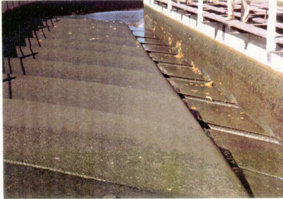
Upstream view of riffle-deflector vortex-tube sand trap installation in supply canal for Colorado Fuel and Iron Co. (Pueblo, Colorado). Capacity equals 250 \text{ ft}^3/\text{s} .
