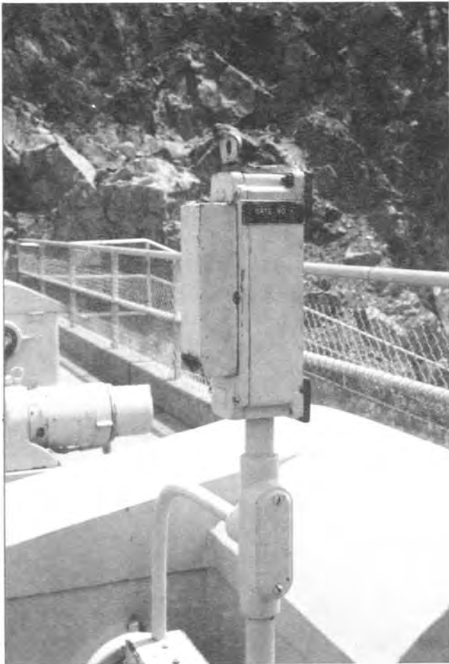
Photo 6.—Small box attached over pushbuttons.
