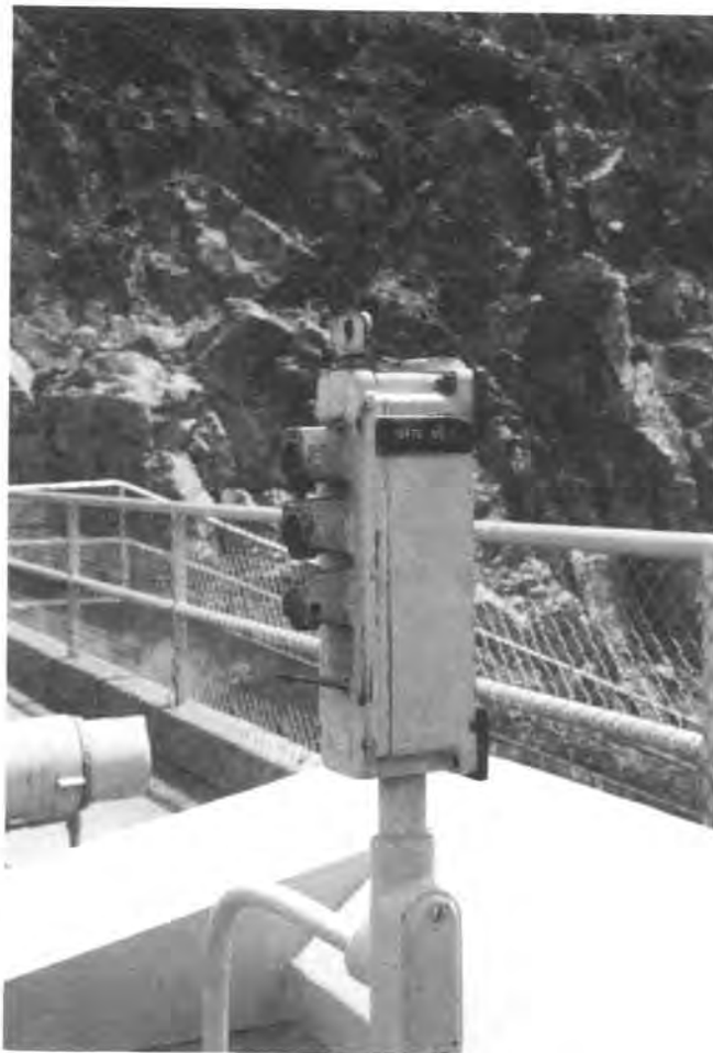
Photo 5.—Spillway gate pushbutton control.
