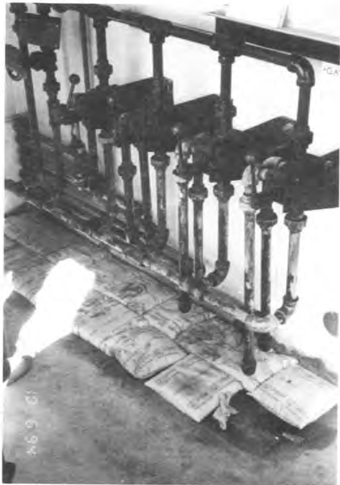
Photo 8.—Square pig absorbents placed beneath hydraulic controls in Unity Dam outlet works control house.
