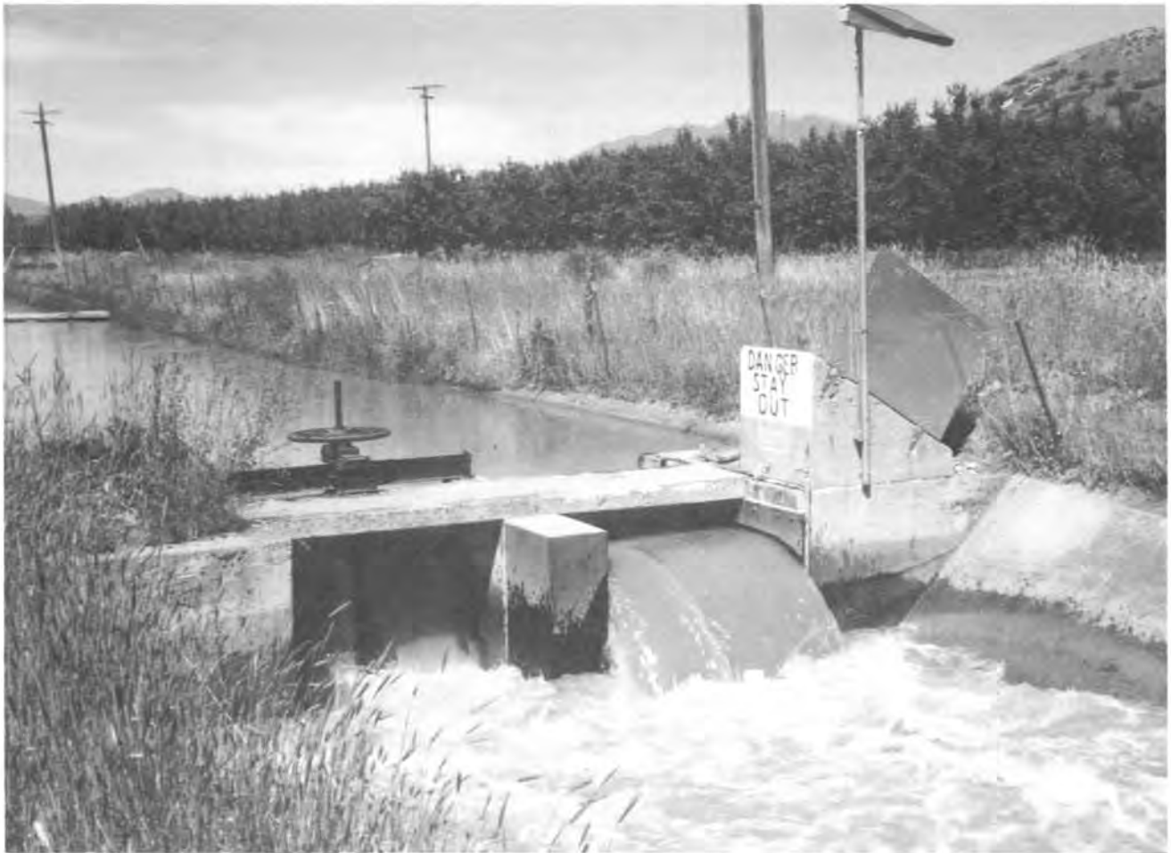
Photo 4.—The rehabilitated check structure with flow over the inflatable gate. The control system hardware is installed in the vault on the far side of the canal.
