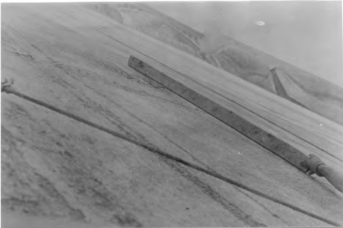
Figure 1. Spillway, Grand Coulee Dam, showing "humped" concrete surface and cavitation erosion.
