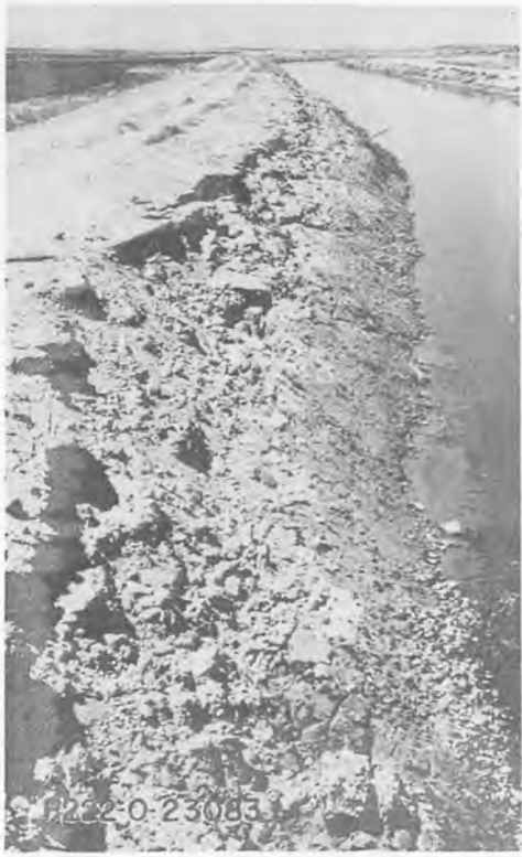
(b) Closeup Of Bank Failure
