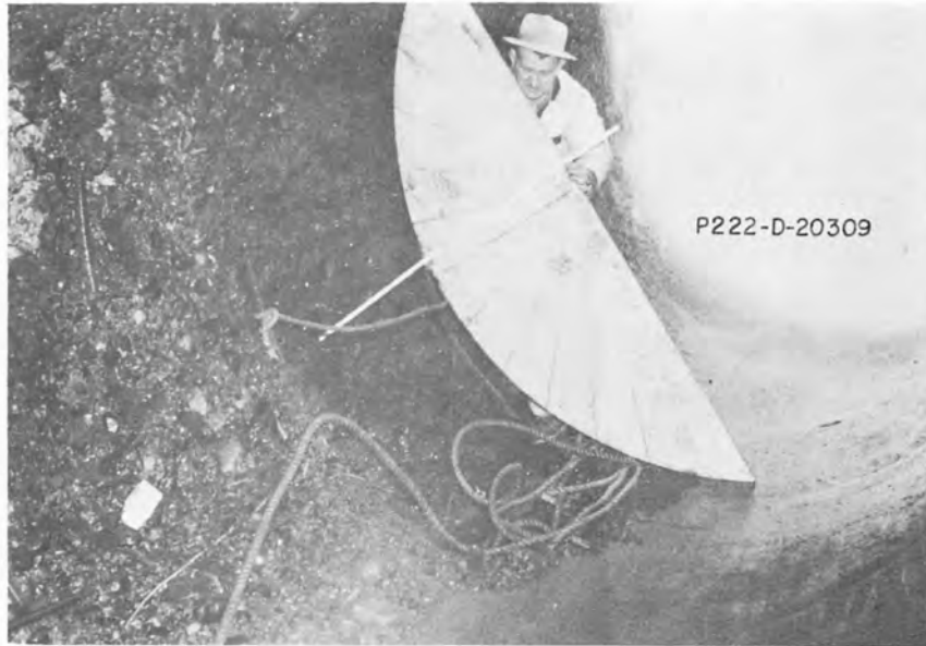
Figure 9--Severe cavitation-erosion in concrete exit trough downstream from liner cone--Grand Coulee Dam Outlet.
