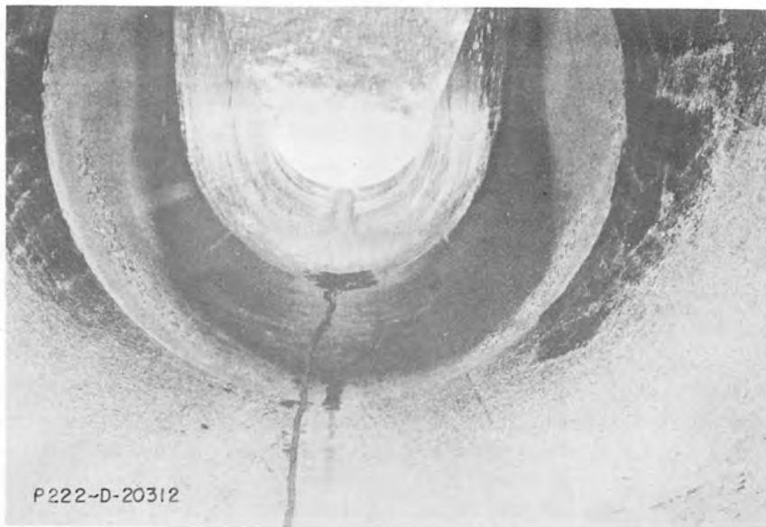
Figure 10--Typical early-stage cavitation-erosion in walls of concrete exit trough downstream from liner cone--Grand Coulee Dam Outlet.
