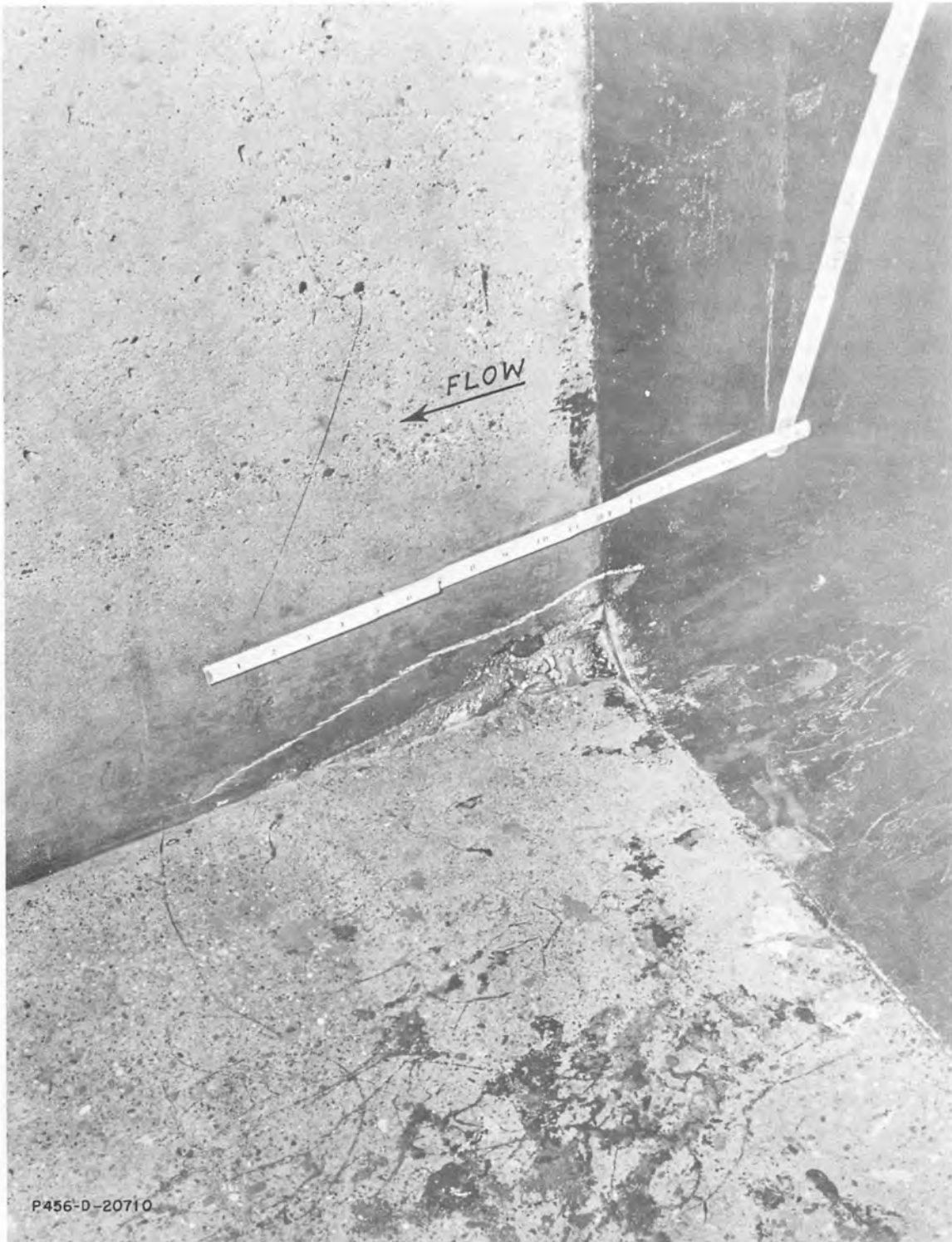
Figure 6--Slight cavitation-erosion, slope away from flow at fillet downstream from outlet gate frame--Palisades Dam.
