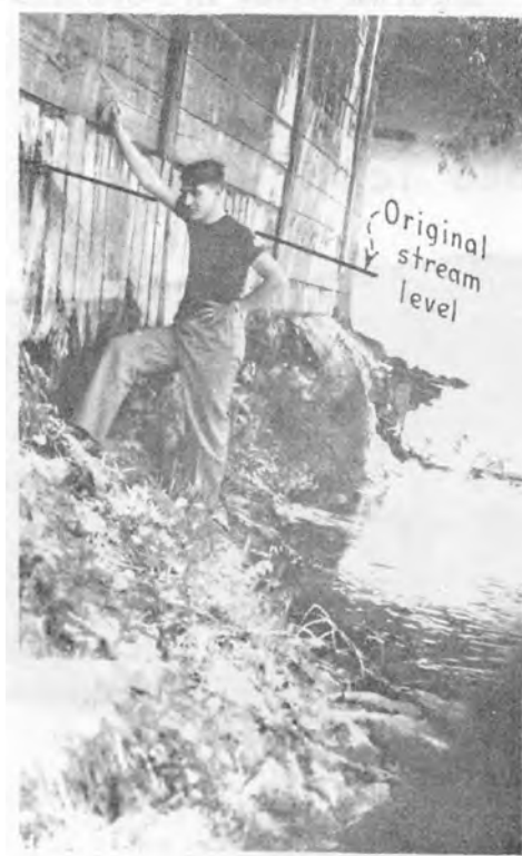
Figure 5. Bed Lowering in Cherry Creek, Denver, Colorado, Caused by Reduction of Sediment Load
