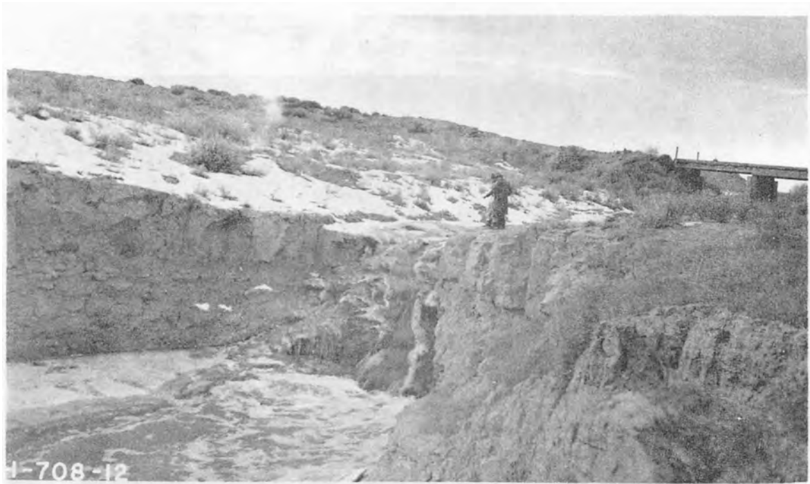
Figure 4. Waterfall on Five Mile Creek, Wyoming, Resulting from Grade Reduction Caused by Increase in Discharge
