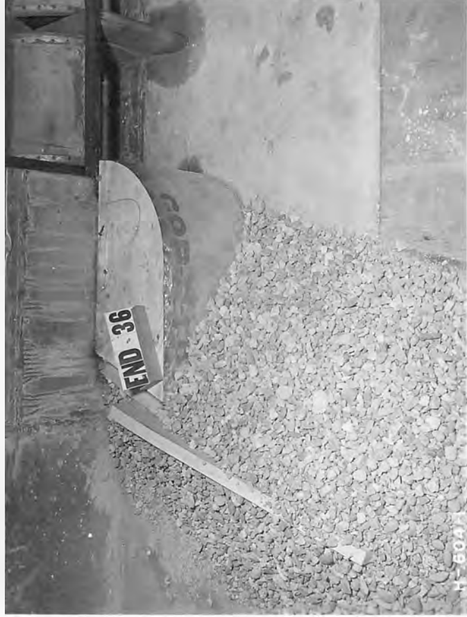
A. Ripped dike upstream from left training wall nose, no flow
