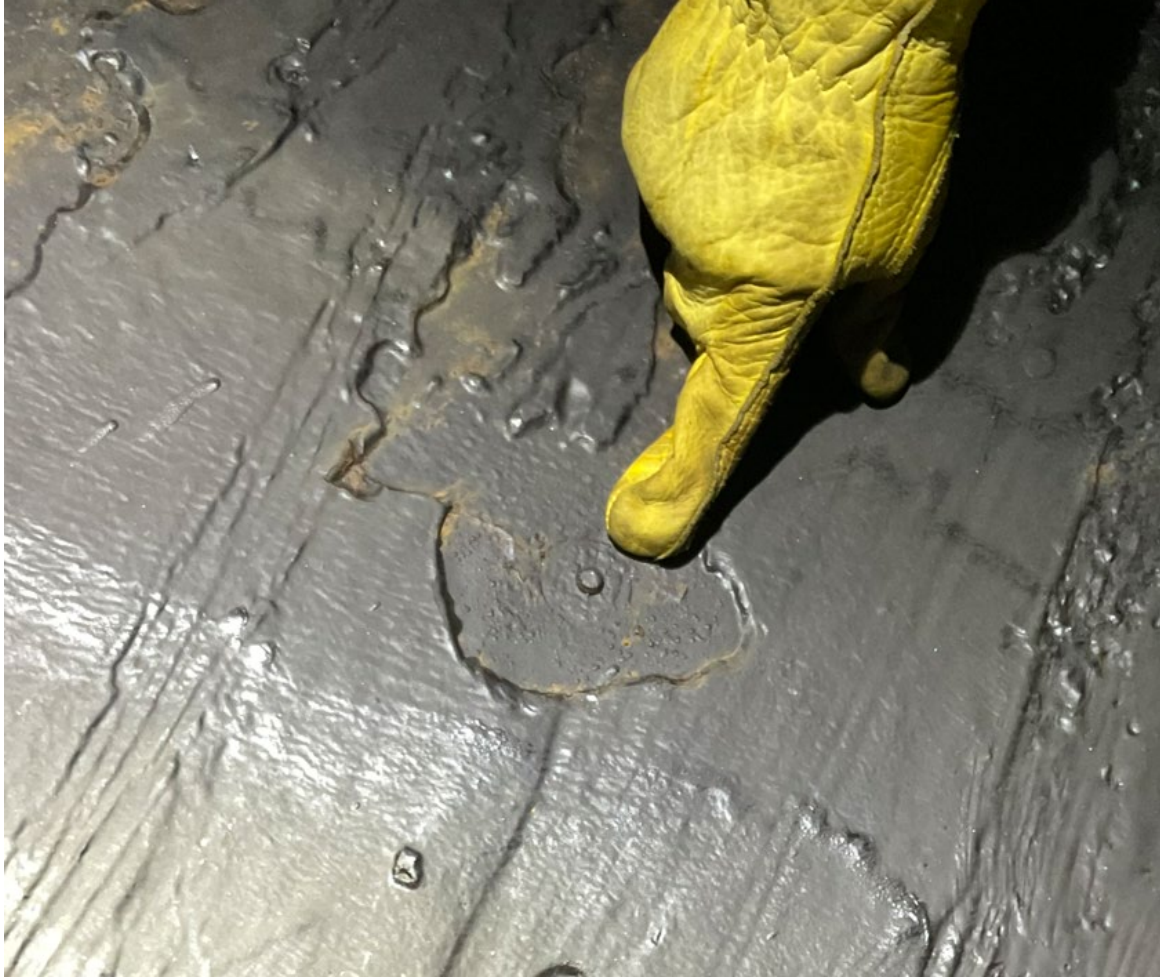
Figure 4. Example of a pressure tap that has been covered by a repair coating.
