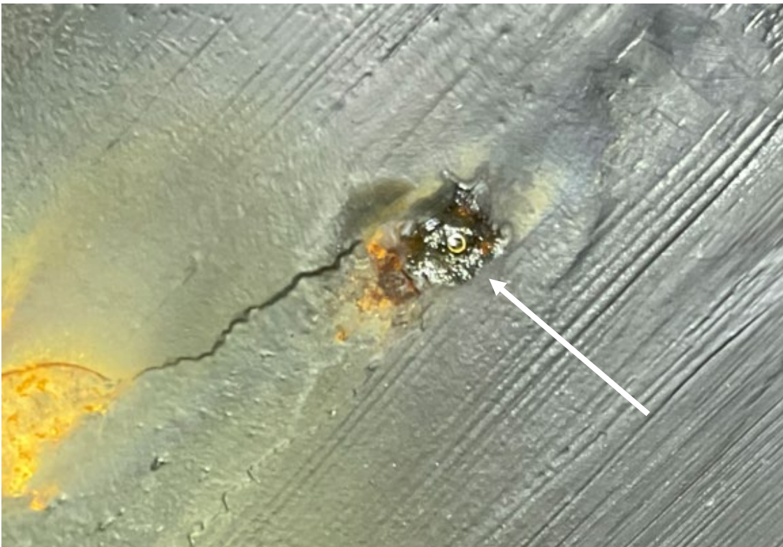
Figure 3. Example of a pressure tap with corrosion and coating loss causing surface irregularities near the tap.
