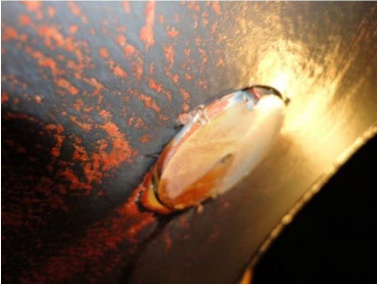
Figure 2. Example of a pressure tap insert that protrudes inside the pipe wall causing an offset.
