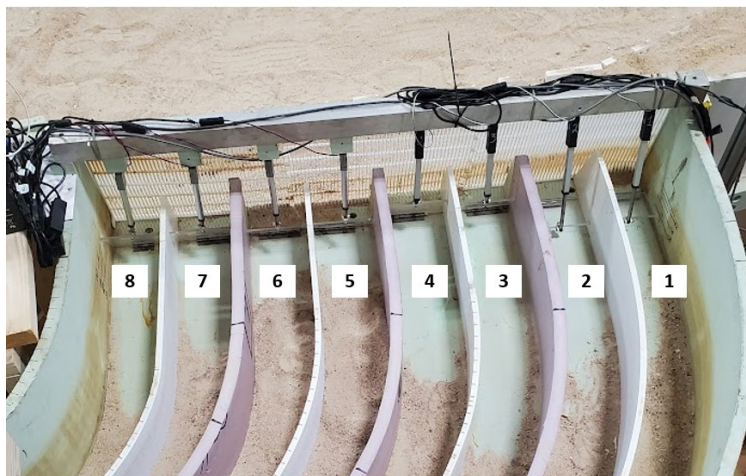
Figure 8. Added canal intake gates (looking upstream toward intake) with individual actuators installed to adjust gate settings remotely.
