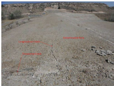
13. Transverse crack (foreground) in dam crest at STA 6+50 in foreground, looking left. Longitudinal crack extends from transverse crack about 20 feet to left. Top lift is unbonded left of transverse crack and downstream of longitudinal crack.
