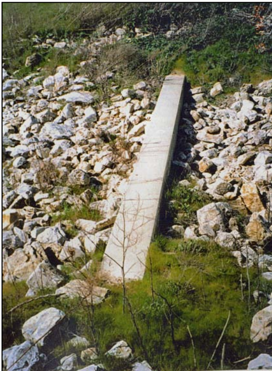
Figure 1.5.1.3-2. Example: Emergency spillway (grade control sill), San Justo Dam, California.
