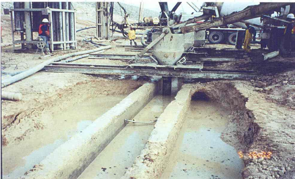
Figure 16.2-3. Guidewall and tremie backfill placement of SCB into the trench (Twin Buttes Dam, Texas).
