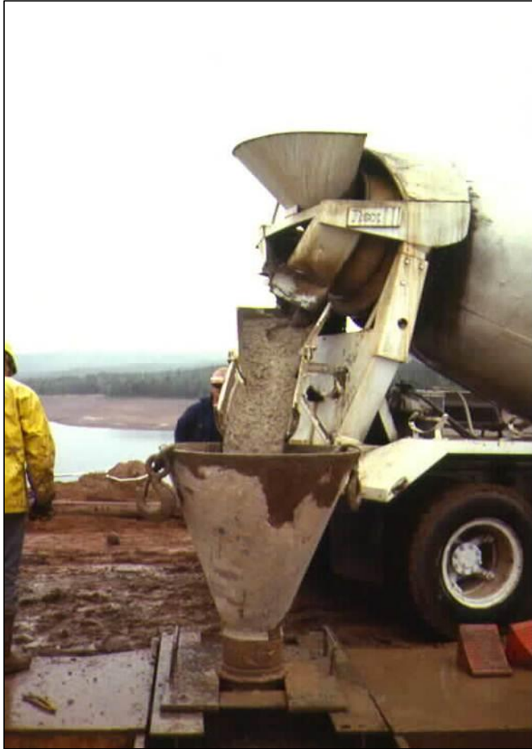
Figure 16.7.13-1. Tremie concrete placement in a concrete cutoff wall (Meeks Cabin Dam, Utah).
