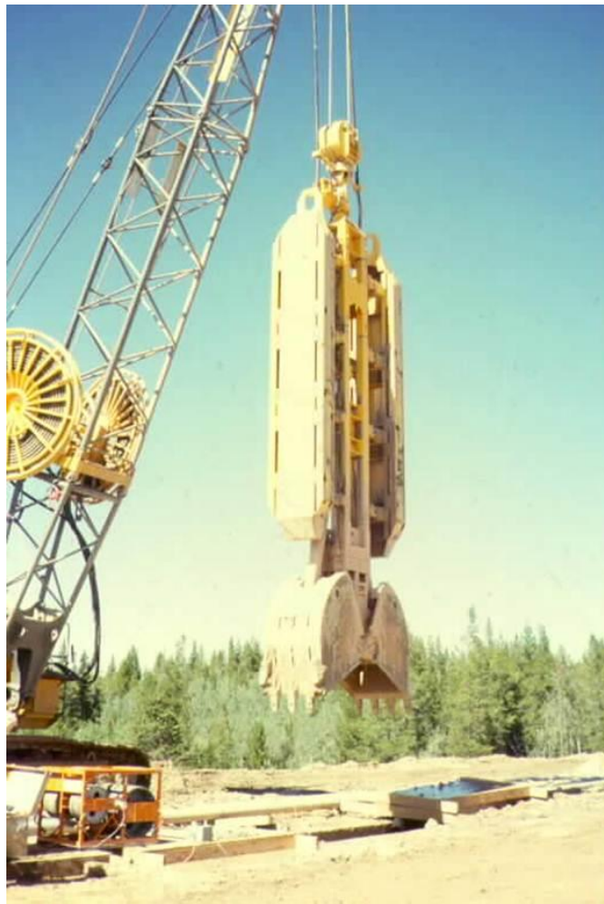
Figure 16.7.4-1. Clamshell excavation of portions of plastic concrete cutoff wall (Meeks Cabin Dam, Utah).
