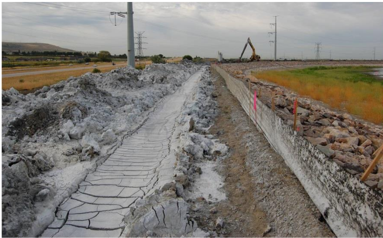
Figure 16.5.5-3. CB cutoff wall after initial set (showing cracking) (A.V. Watkins Dam, Utah).
