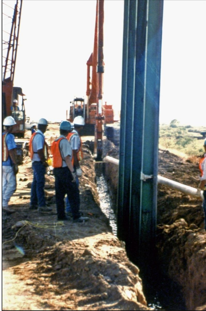
Figure 16.8.3-3. Installation of geomembrane cutoff wall into biopolymer slurry trench (Reach 11 Dikes, Arizona).
