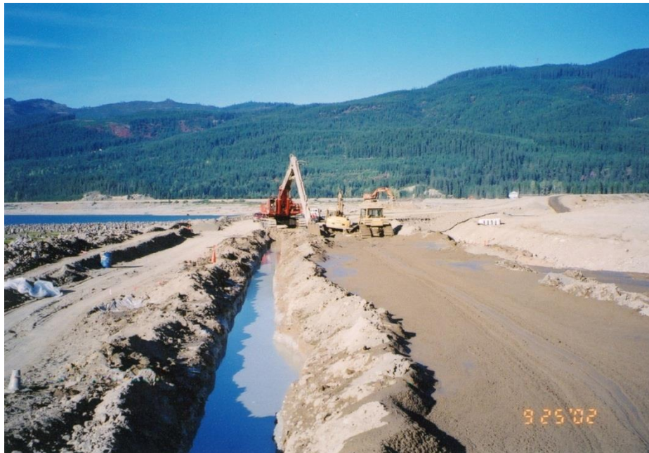
Figure 16.4.7-2 SB backfill being mixed with bentonite slurry adjacent to the trench at Keechelus Dam, Washington.
