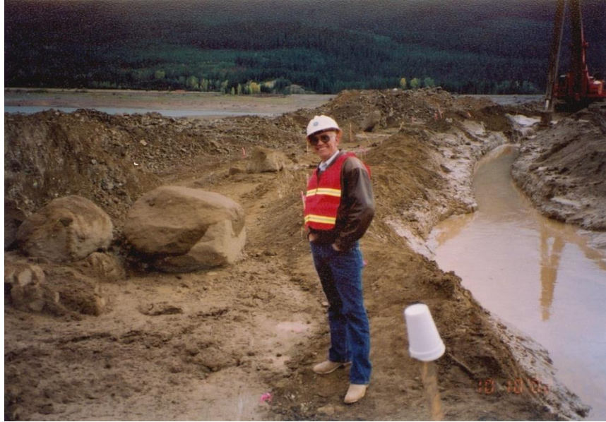
Figure 16.4.7-1 Large embedded boulders removed from SB cutoff wall at Keechelus Dam, Washington.
