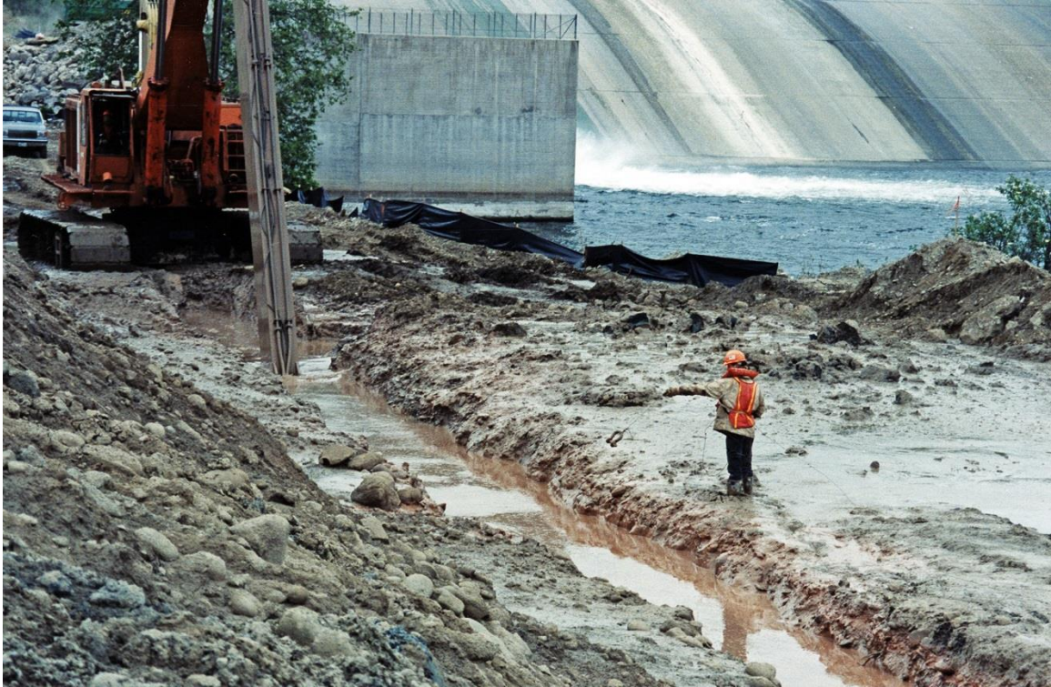
Figure 16.4-1. Excavation of SB cutoff wall using extended reach backhoe. Note inspector using weighted tape to measure depth (Bradbury Dam, California).
