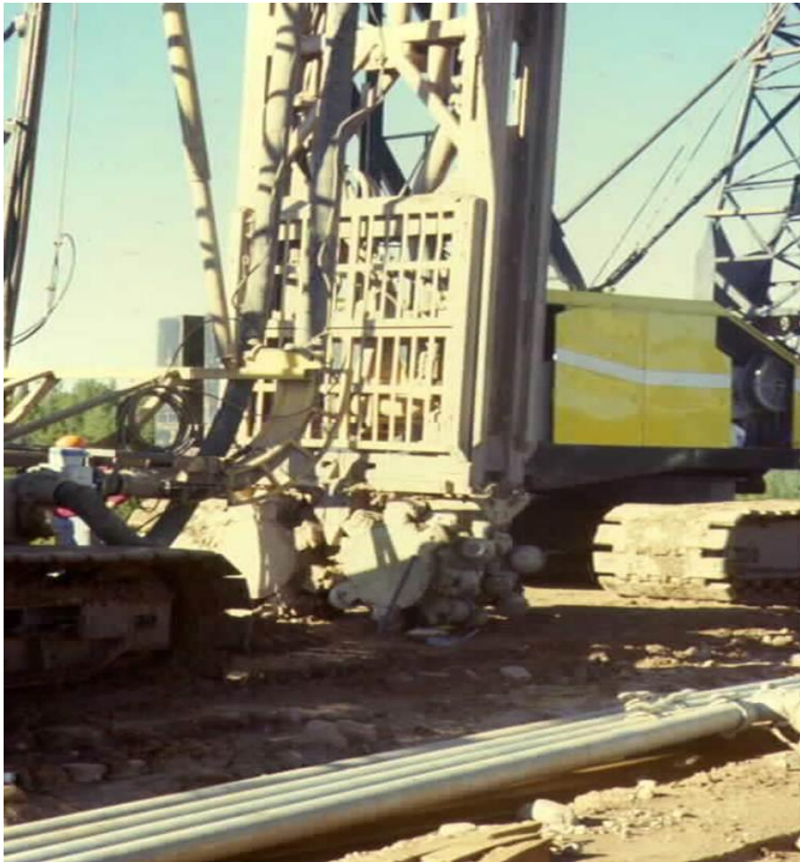
Figure 16.7.4-2. Rock mill used to excavate portions of plastic concrete cutoff wall (Meeks Cabin Dam, Utah).
