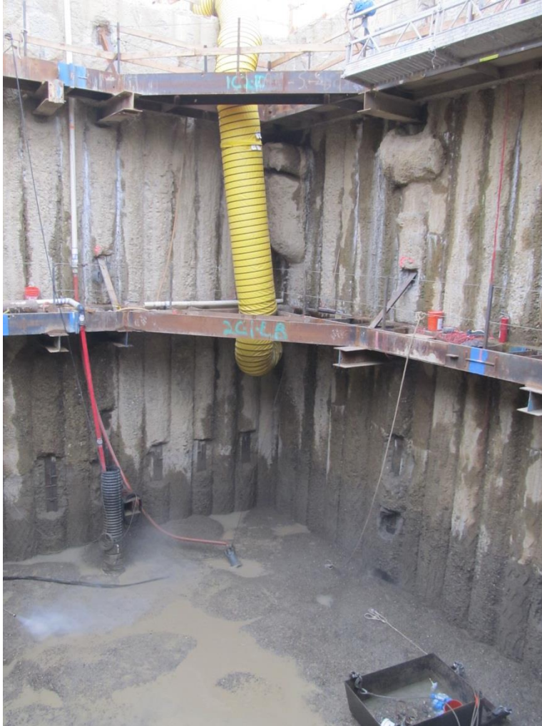
Figure 16.10.2-2. Secant piles exposed in the wall key block excavation showing exposed steel wide flange reinforcement (Mormon Island Auxiliary Dam, California).
