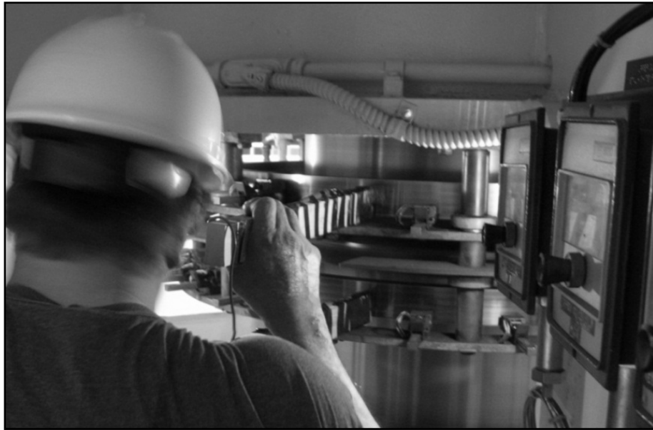
Figure 1.5.7.3-1. Heat run test (section 1.5.7.3). Carbon brushes mounted to dry wooden sticks are held against the field collector rings for voltage measurement to determine field resistance.
