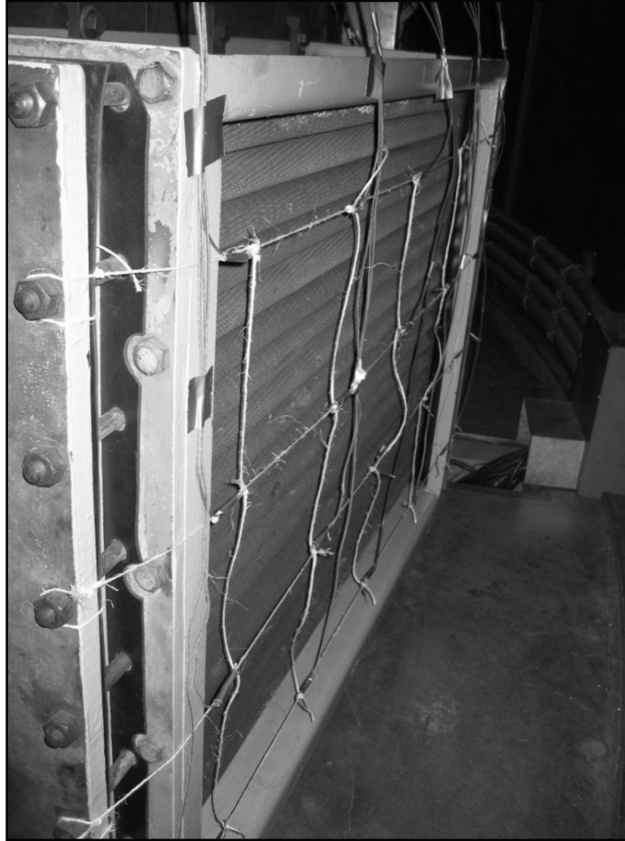
Figure 1.5.7.2-1. Trial heat run test (section 1.5.7.2). Photograph showing placement of 20 thermocouples at the cold air discharge face of an air cooler inside the stator air housing.
