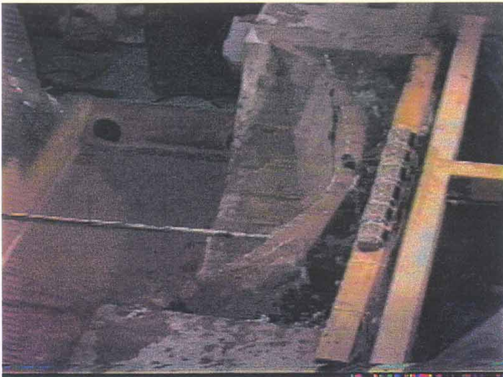
Model M8 -- 6/21/00 North view, initial cracking
