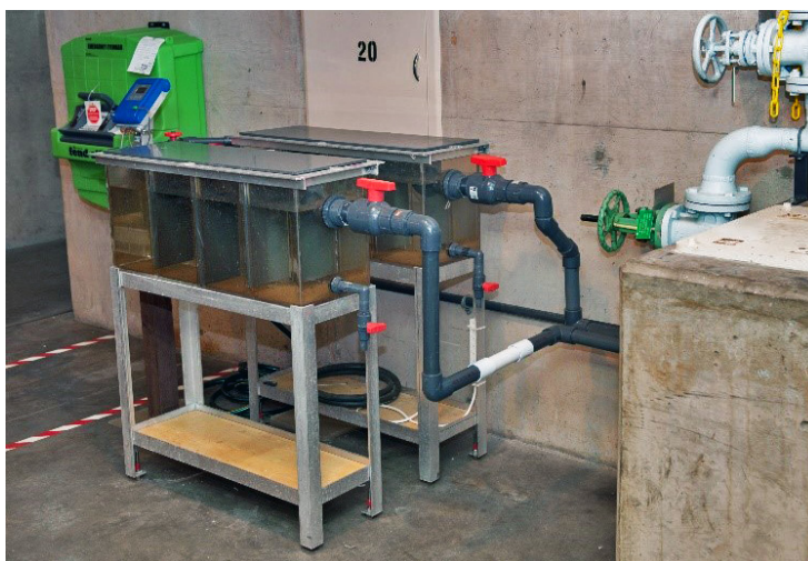
The effectiveness of copper treatments at preventing invasive mussel settlement in pipes will be analyzed using bio-boxes similar to those installed at Davis Dam.
