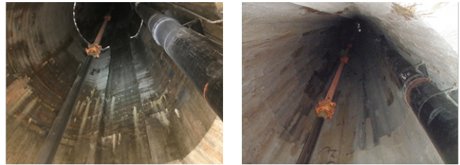
Headgate shaft at Trinity Dam. Photo at left is before the EOP system was installed and the photo at right is after 12 months showing the system is reducing the water leakage.
