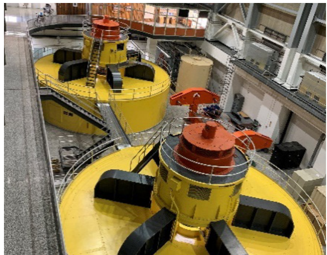
New Online Monitoring Glen Canyon Unit 1 and Unit 2, the test units for the pilot system.
