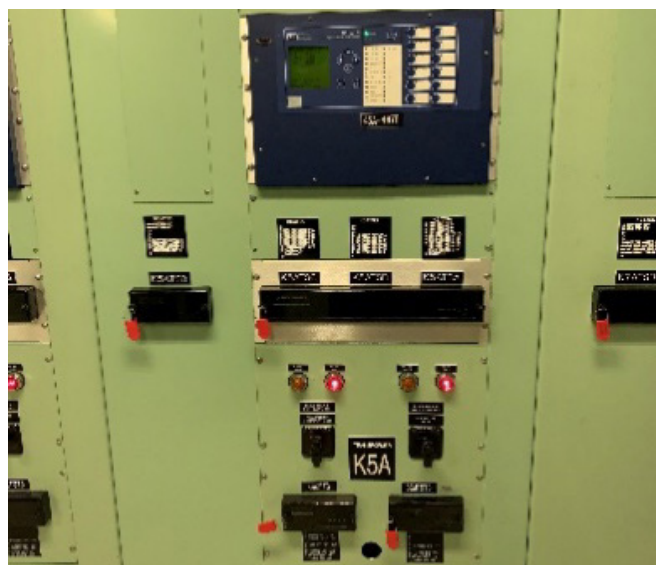
Transformer Differential Relay, the relay will be connected to the pilot system.
