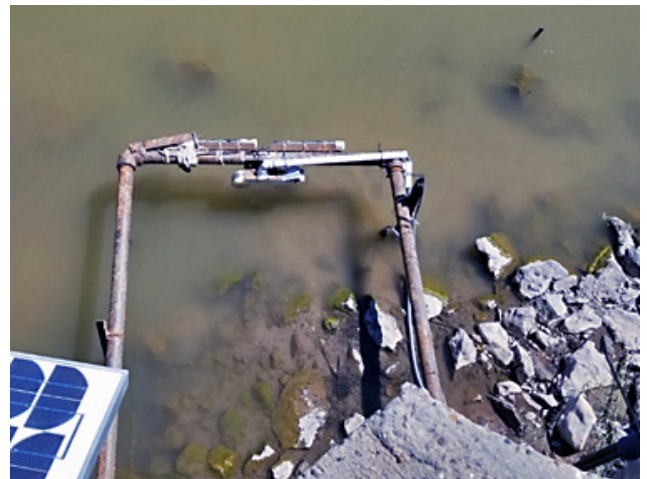
Photo of mounting structure and acoustic instruments after installation at low water.
