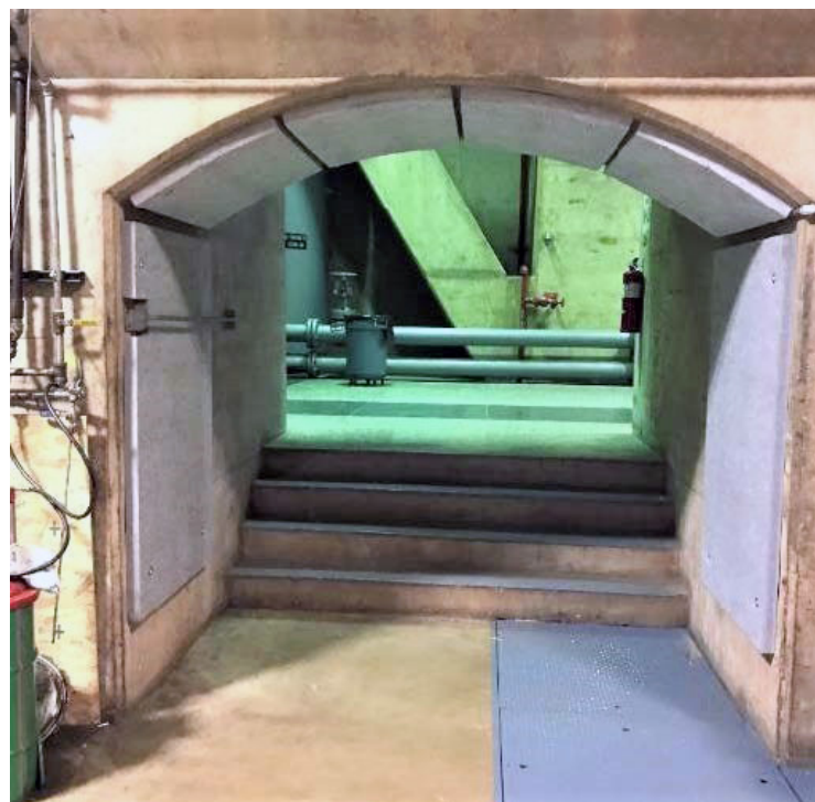
Acoustic absorption panels installed in the opening between two galleries at Hoover Powerplant.
