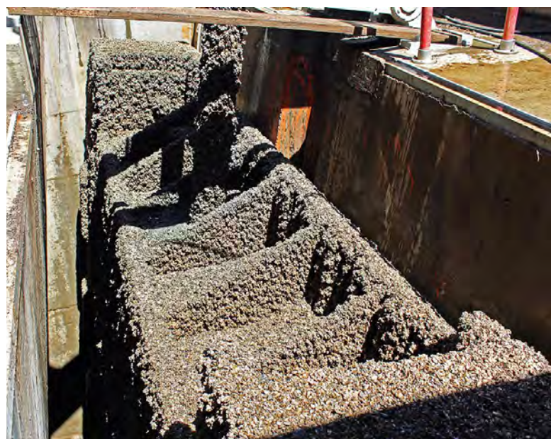
Quagga mussel fouling on a fixed wheel gate at Glen Canyon Dam.
