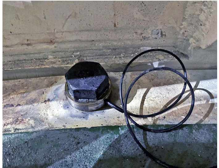
'Smart' washers installed on this turbine head cover bolt allow for continual real time monitoring of bolt tightness and load.
