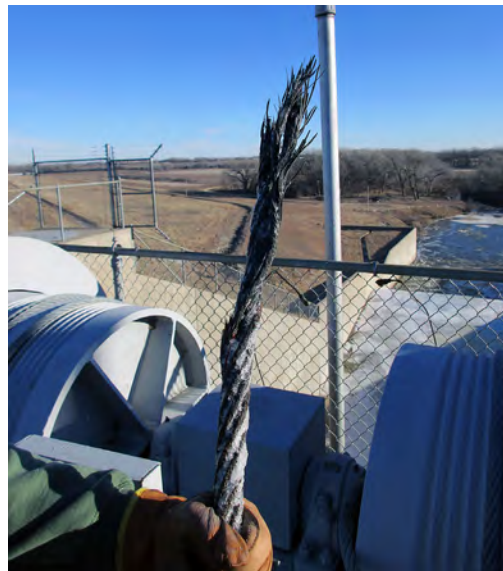
Example of a catastrophic wire rope break.
