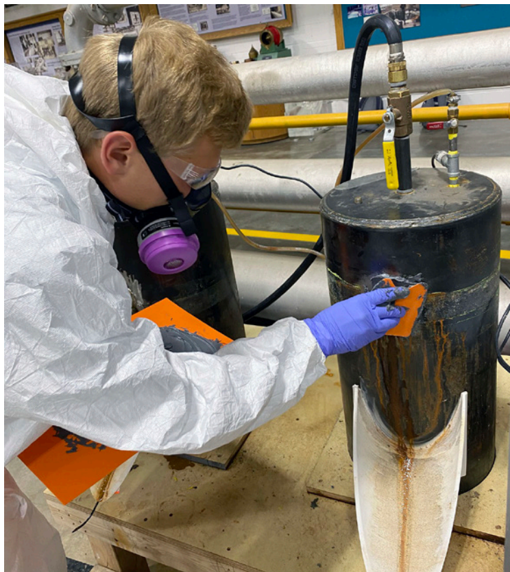
Researcher wearing personal protective equipment applying an epoxy repair to the laboratory pipe set-up.
