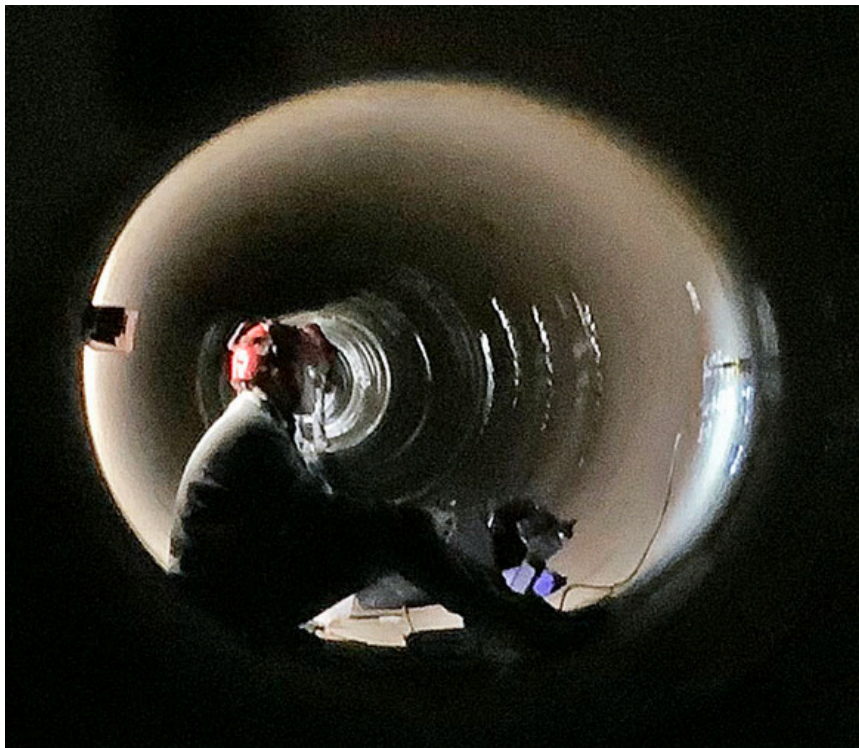
Reclamation inspector collects EIS data from inside of Collbran Salt Creek Siphon.
