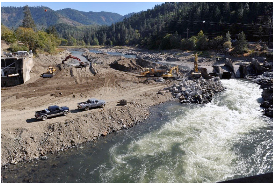
Looking upstream at Savage Rapids Dam removal in Oregon during construction. (Photo credit Jennifer Bountry)
