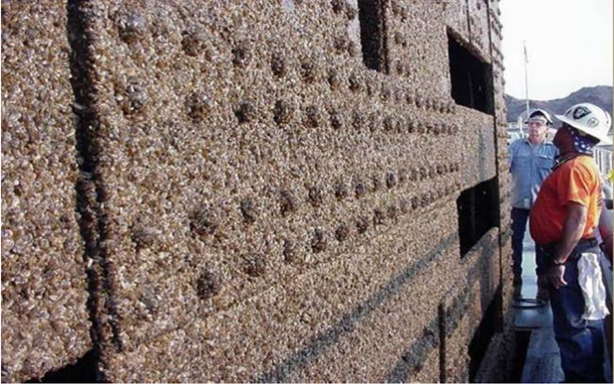
Figure 9. Invasive Quagga mussels on bulkhead gate. Photograph courtesy Denise Hosler, Reclamation.
