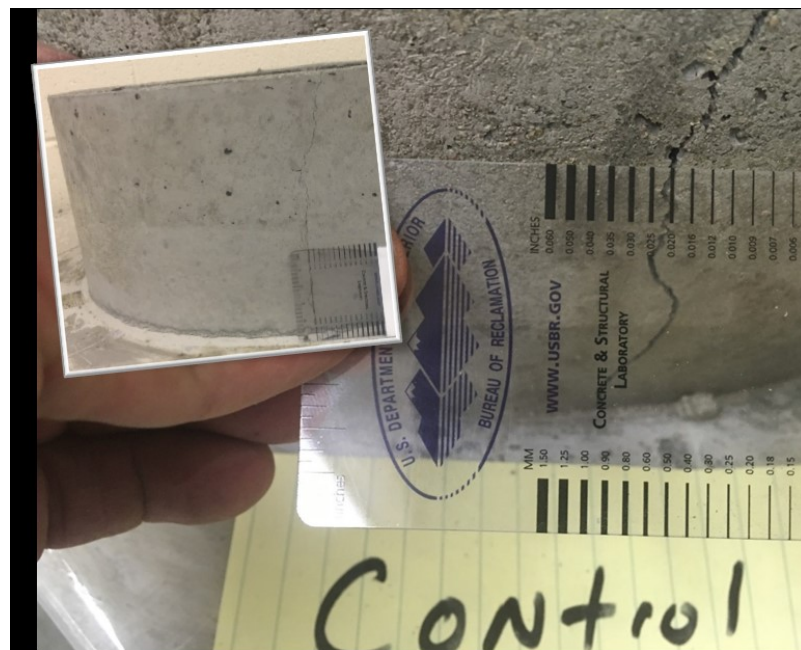
Restrained shrinkage tests on modern admixtures show decrease in crack width and a greater time to cracking.
