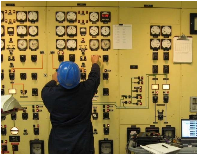
Reclamation plant operator starting a hydro generator.
