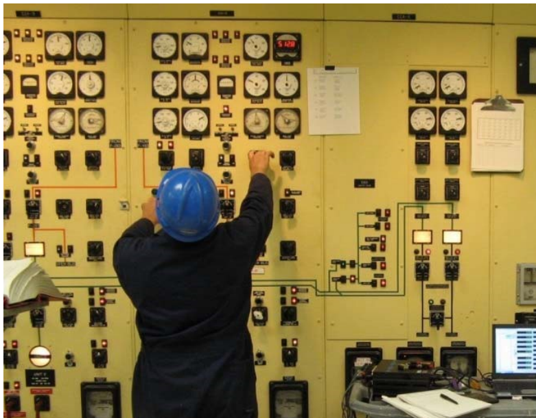
Reclamation plant operator starting a hydro generator.
