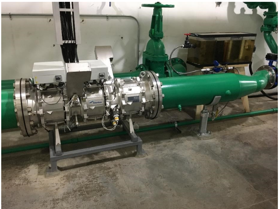
HOD UV unit installed at Parker Dam for reduction of biofouling the generator cooling systems.
