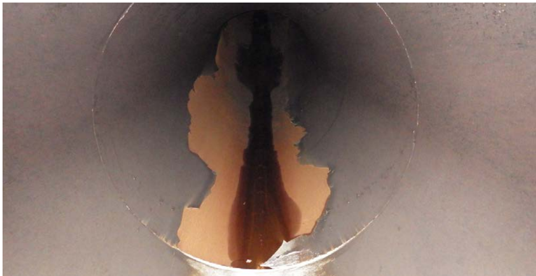
Figure 2: Delaminated elastomeric polyurethane lining in the Unit 2 penstock at Flatiron Penstocks.
