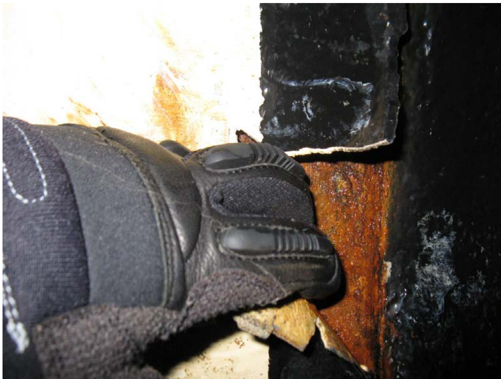
Figure 6: Polyurethane termination point near a jet valve. Cracking and subsequent corrosion undercutting caused the lining to disbond and lift off the pipe surface.
