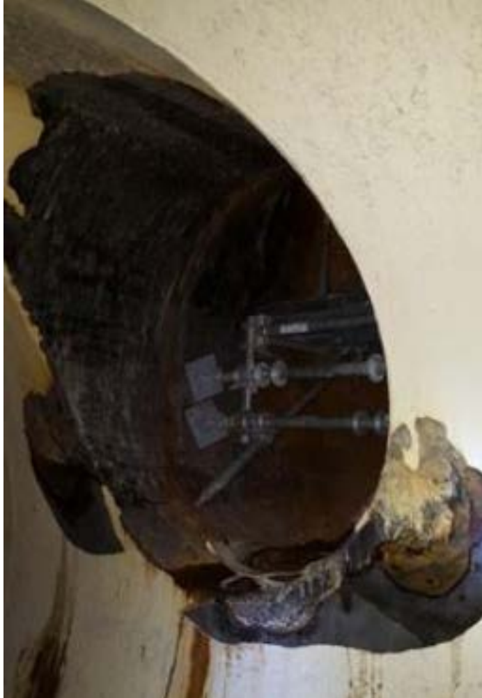
Figure 4: Damaged lining around a manhole at Enders Dam after one year of service.
