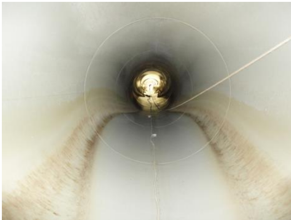
Figure 9: General condition of an epoxy lining after one year of service in the outlet works at Shadehill Dam.
