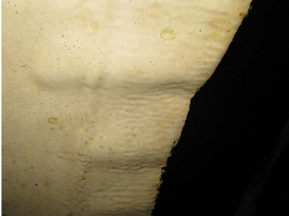
Figure 5: One area of disbonded elastomeric polyurethane in the outlet works at Enders Dam [7]. Disbonded polyurethane was found after one and six years of service.
