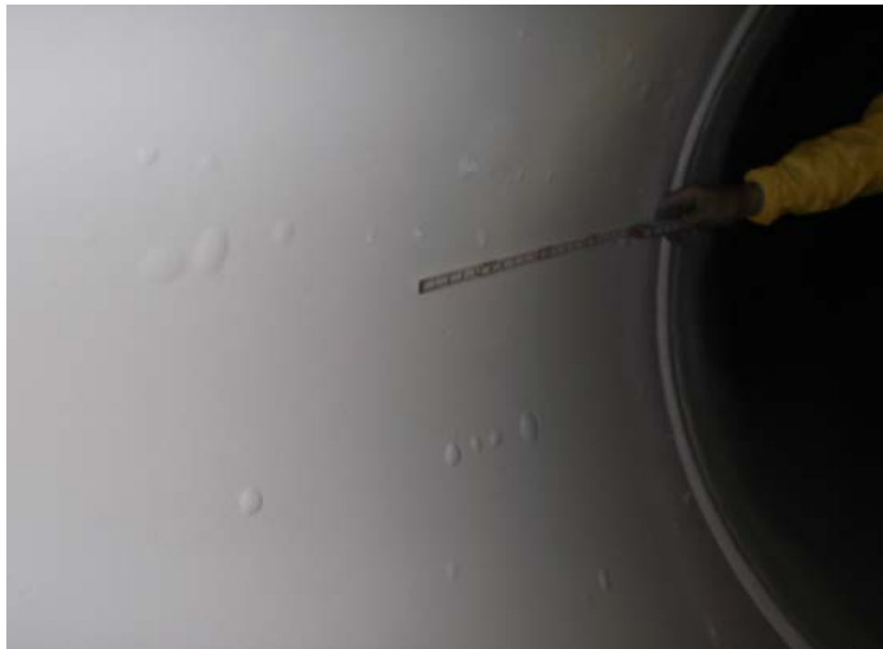
Figure 3: Extensive blistering shortly after the application of a fast set polyurethane lining caused by a heat-sink phenomenon. Flatiron Penstocks, 2017.
