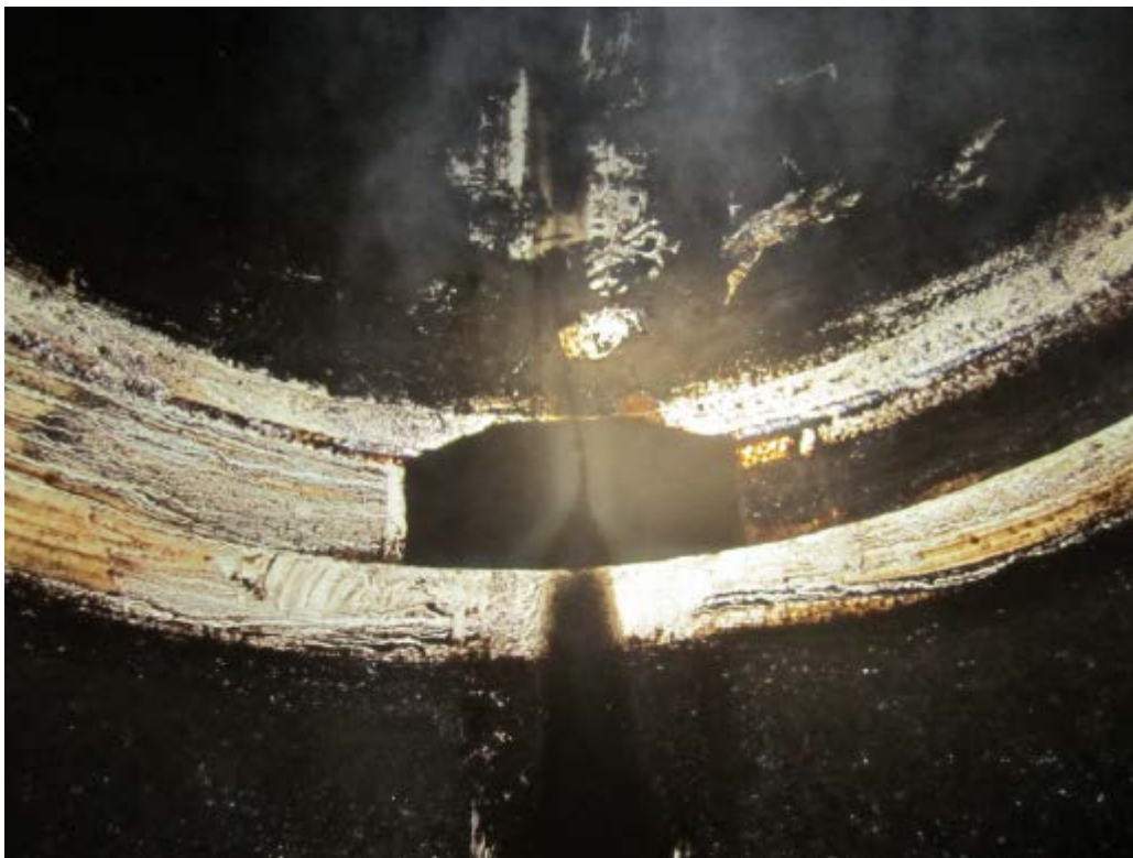
Figure 7: Typical coating condition at an expansion joint in the outlet works at Platoro Dam. The polyurethane lining had been in service for five years.
