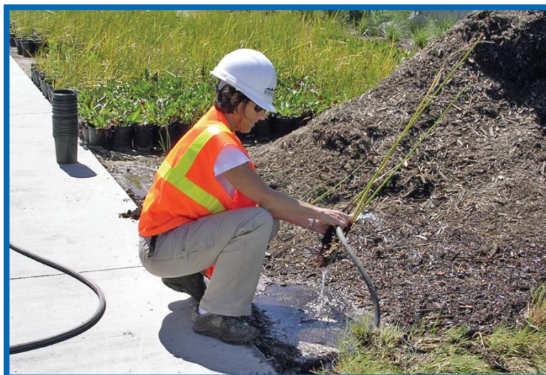
Building saline wetlands at the administrative building in Oxnard, California. (see next page for the final ponds)
